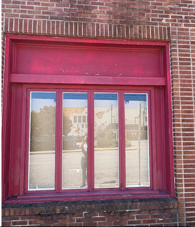
Easternmost infilled windows. Proposal will remove entire window and trim unit and replace with aluminum windows.
