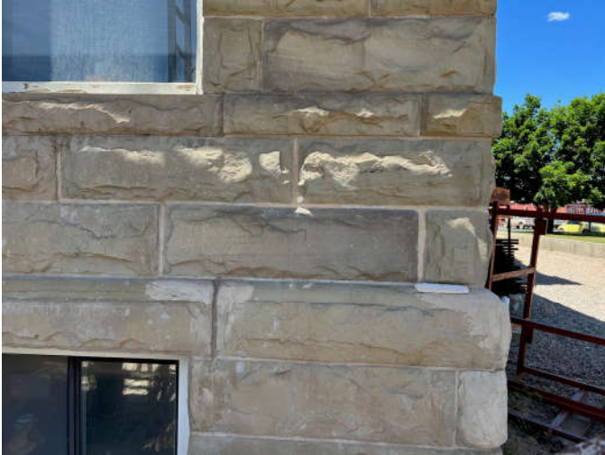
Photo #3: An area of the east wall was used for two mortar pointing samples. The mortar approved for the tower was selected.
