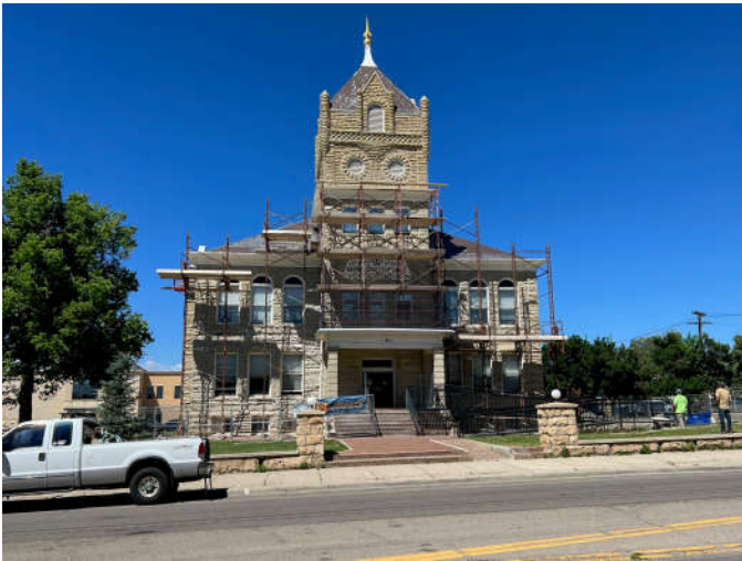
Photo #1: Scaffolding was erected to allow the masons access to all areas of the east elevation. The front entry remains open to the public.
