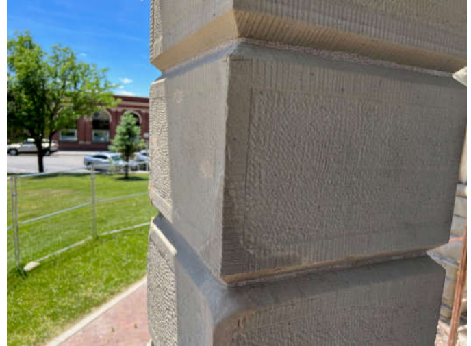
Photo #5: A corner of the entry porch column was patched with the tooling approved. Jahn mortar matching the stone will be provided.
