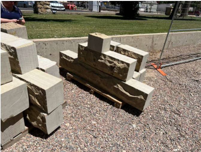
Photo #4: A load of replacement stones was delivered to the site. The large lintel stone at the bottom of the pile is cracked along one of the bedding planes.
