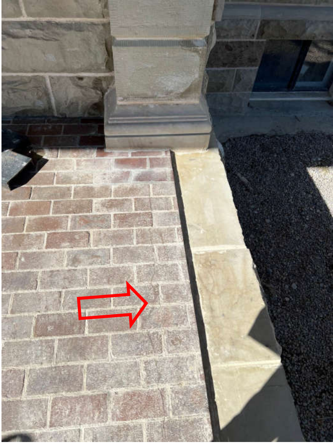
Photo #6: The new guardrails will be installed in the brick pavers rather than the new stone. A crack in the brick pavers was observed. Brick pavers were patched around the pilaster base.
