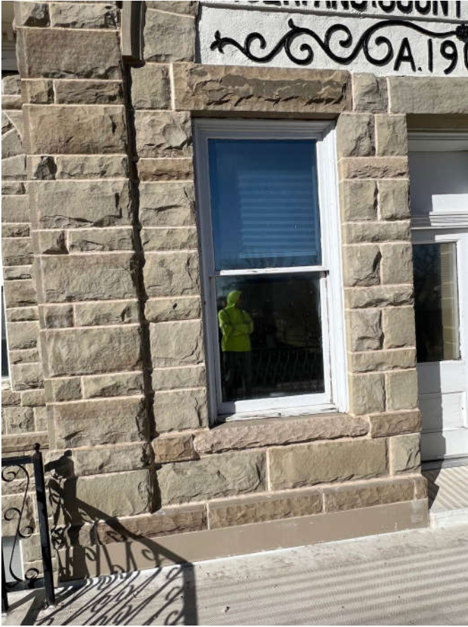
Photo #5: Replacement stone, both above and below the window, was installed along with metal counter flashing at the east balcony wall.
