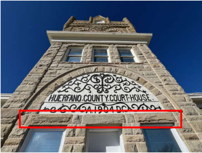
Photo #7: The plaster sign was repaired and repainted. Replacement lintel stones were installed above the second floor windows.
