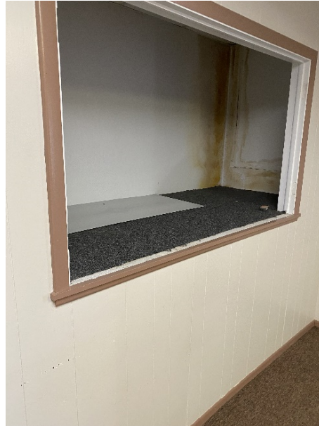
Figure 1: Evidence of water damage
