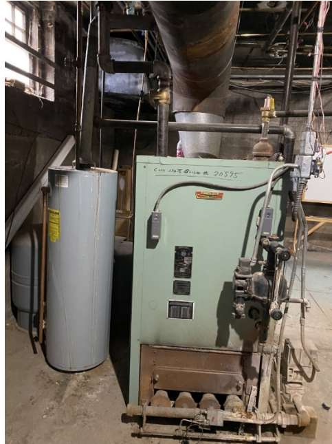
Figure 5: Existing boiler, appears older and may need replacement
