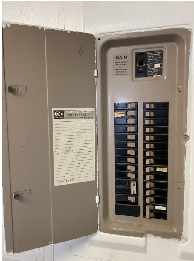
Figure 4: Existing electrical panels, appear older - need to confirm capacity for new use
