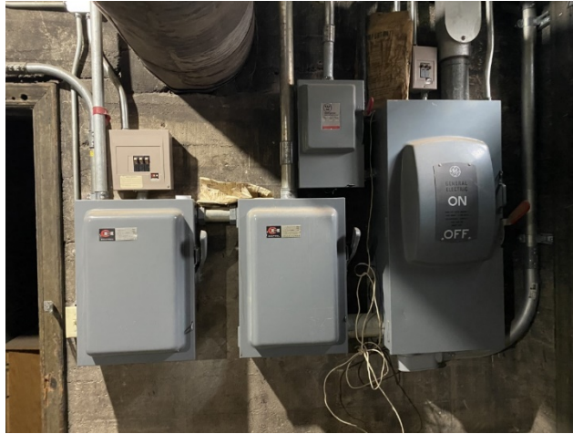
Figure 3: Existing electrical panels, appear older - need to confirm capacity for new use
