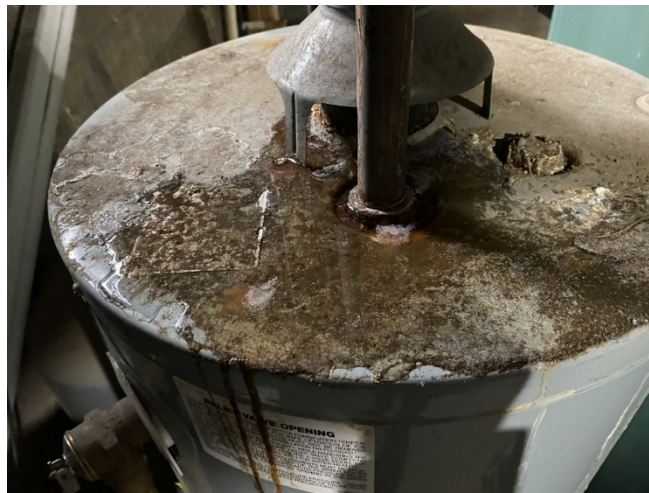
Figure 6: Existing water heater, appears older and may need replacement
