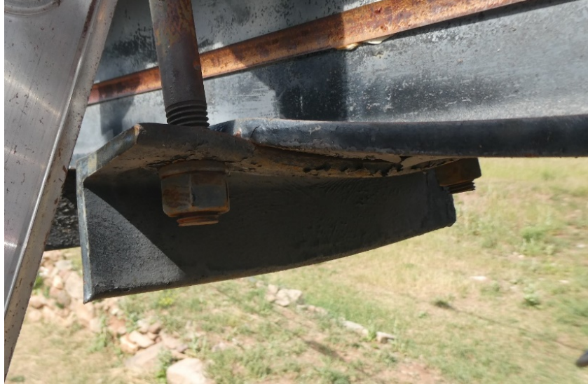
Figure 5 Distorted Support Beam Flanges
