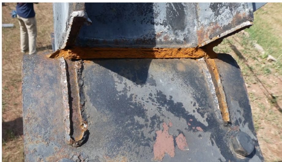
Figure 4 Failed Base Plate Weld Connection
