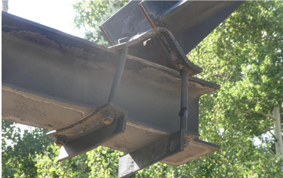
Figure 3 Frame connection Damage
