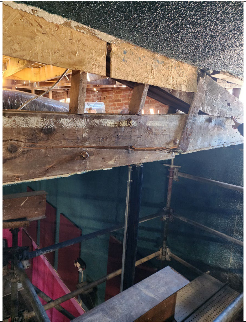
North end of east truss. Split in bottom cord visible following plaster removal.
