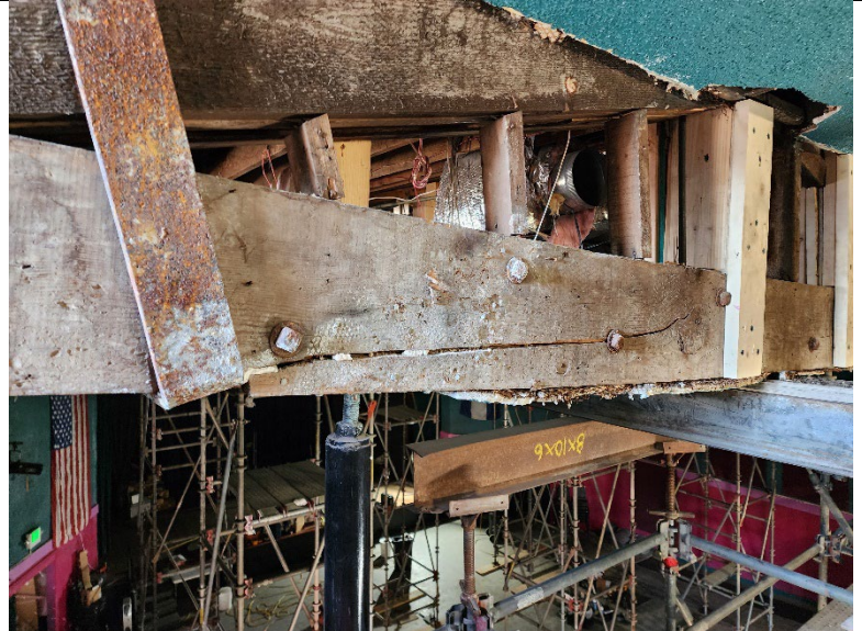
South end of east truss. Split bottom cord visible following plaster removal.
