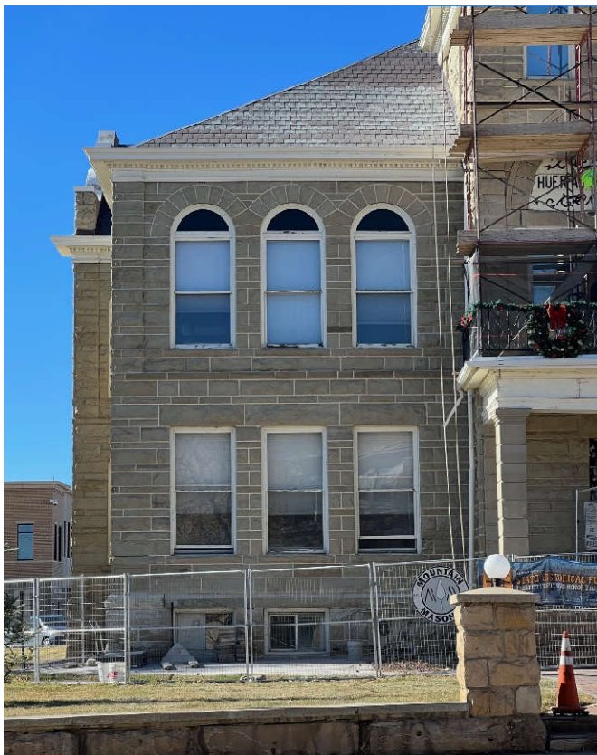
Photo #1: Now that the scaffolding has been removed, work at this end of the wall is now visible.
