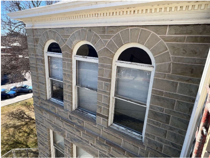
Photo #10: The repointing at the top of the south end of the east wall is completed with the exception of filling two holes below the cornice, which will be accomplished when the boom lift is on site.
