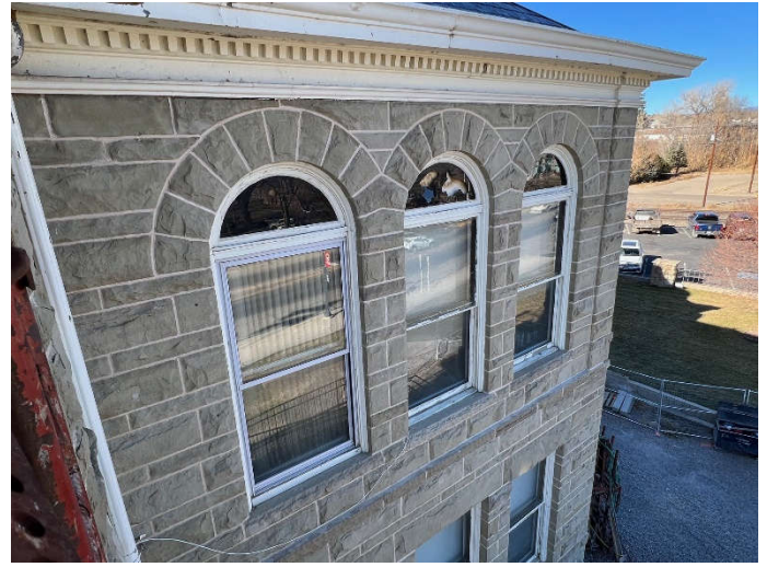
Photo #11: The completed repointing at the top of the north end of the east wall can be seen from the second floor balcony.
