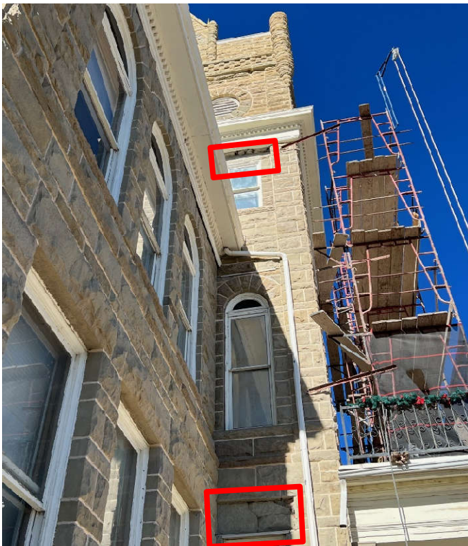
Photo #5: Two lintel stones remain to be installed on the tower's south face.
