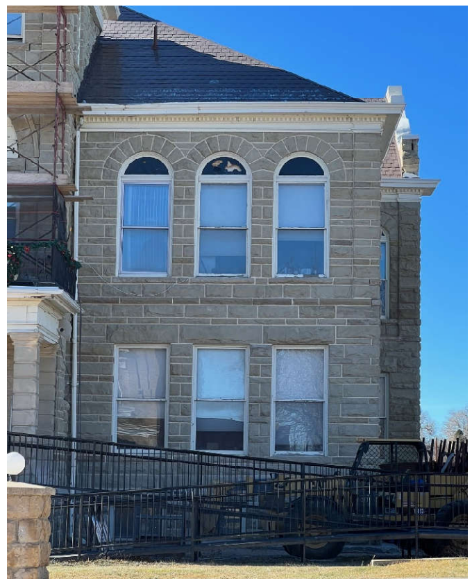
Photo #2: The work at the north end of the east elevation is close to completion with most mortar joints now repointed.
