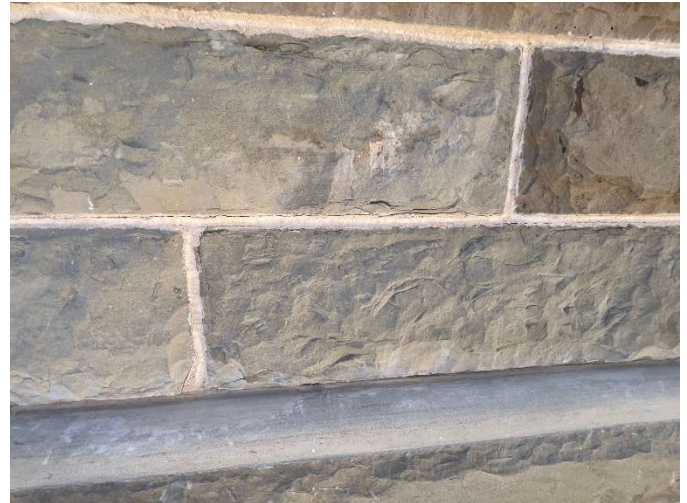
Photo #4: Hairline cracks have developed in some of the repointed mortar joints above the water table stones, which will be repointed.
