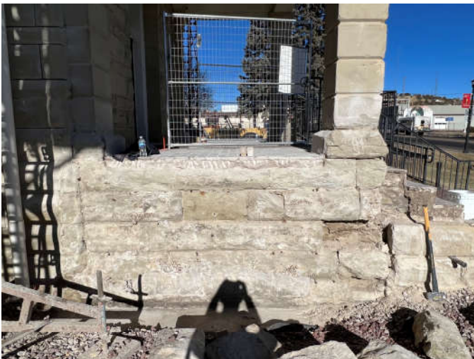
Photo #1: West end of south cheek wall with original sandstone exposed after the outer layer of non-original stone was removed.
