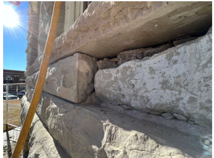
Photo #6: The stone is not thick enough to be refaced so it will be replaced instead.
