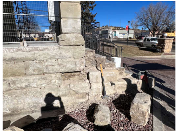
Photo #2: East end of south cheek wall showing deteriorated condition of original sandstone.
