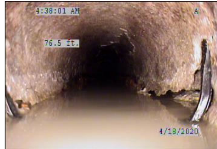
Photo 62: Structural damage (pipe deterioration) (Basin E4).
