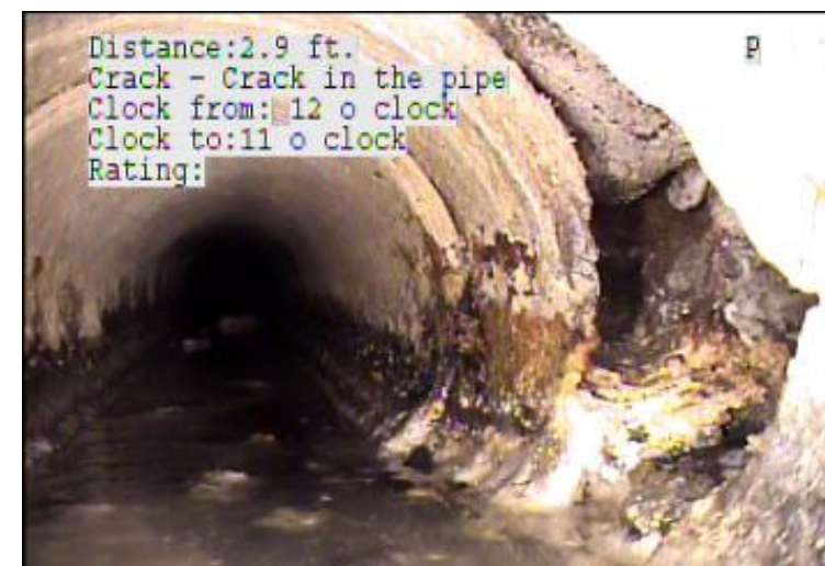
Photo 65: Structural damage (hole in pipe) (Basin E4).
