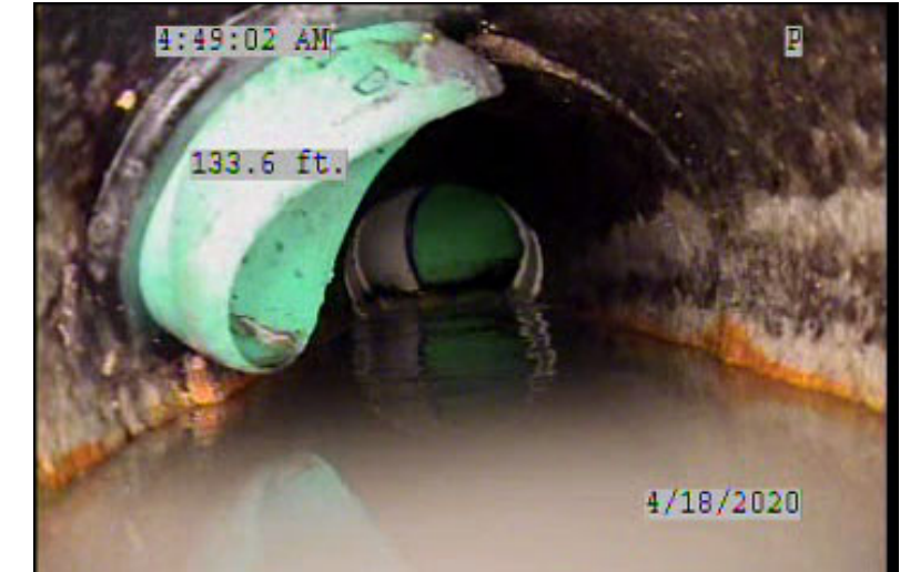
Photo 63: Protruding lateral (Basin E4).
