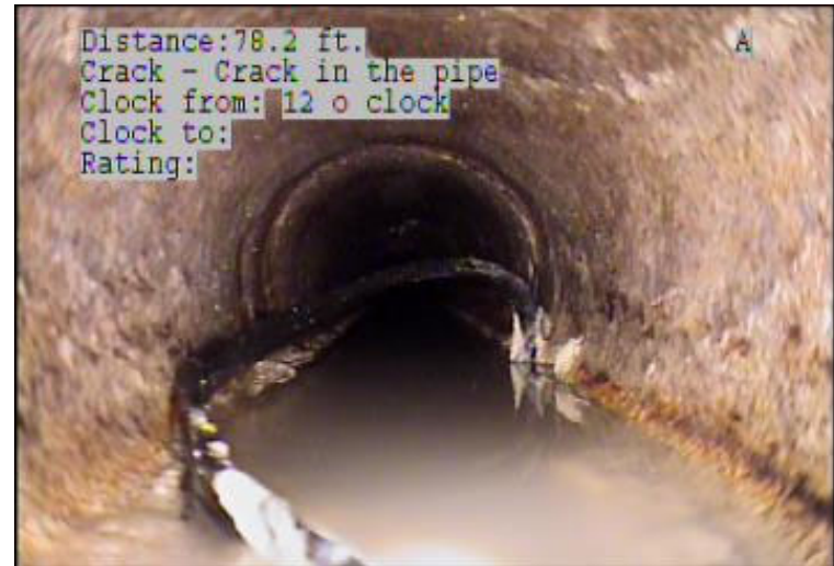
Photo 61: Structural damage (crack in pipe) (Basin E4).
