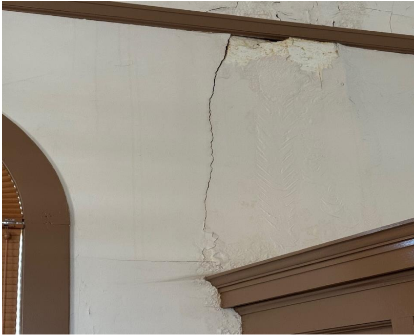
← Water damage at exterior wall @ main entry Photo 1
