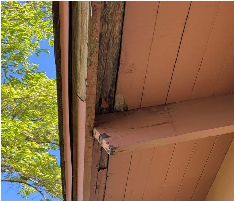
← Water damage @ Existing Eave Photo 5
