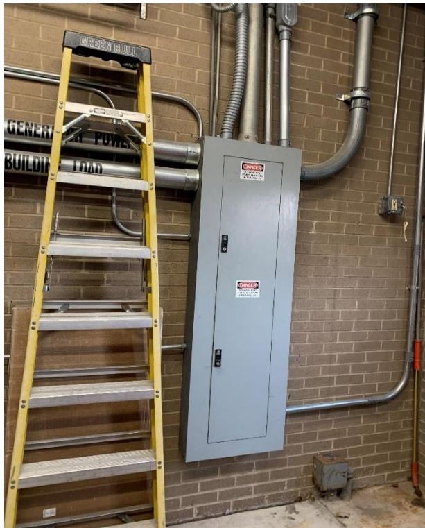
Figure 9 - Generator Distribution Panel
