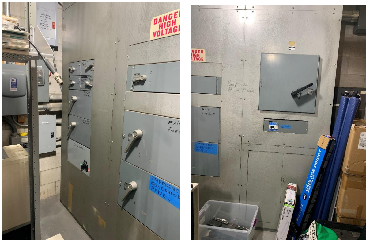
Figure 5 – Police Main Service Switchboard
