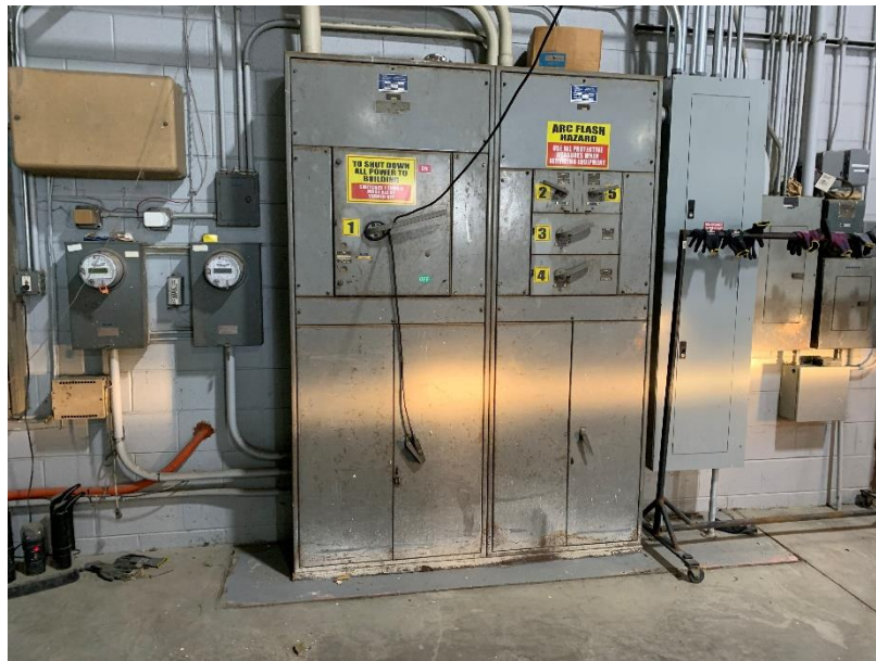
Figure 13 – Public Works Main Service Assembly
