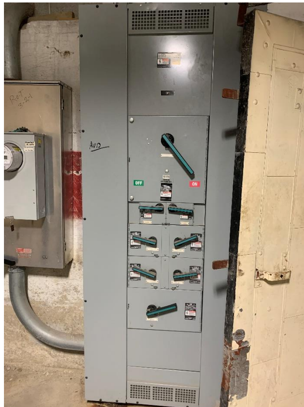
Figure 4 Auditorium Main Service Panel
