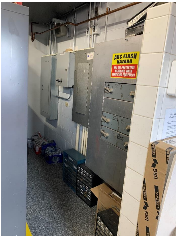
Figure 11 – Fire Dept. Electrical Space
