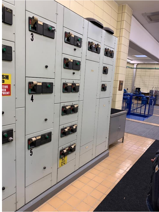
Figure No. 16 – Pump Station No. 1 Main Switchboard
