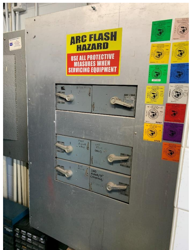
Figure 12 – Fire Dept. Main Service Panel
