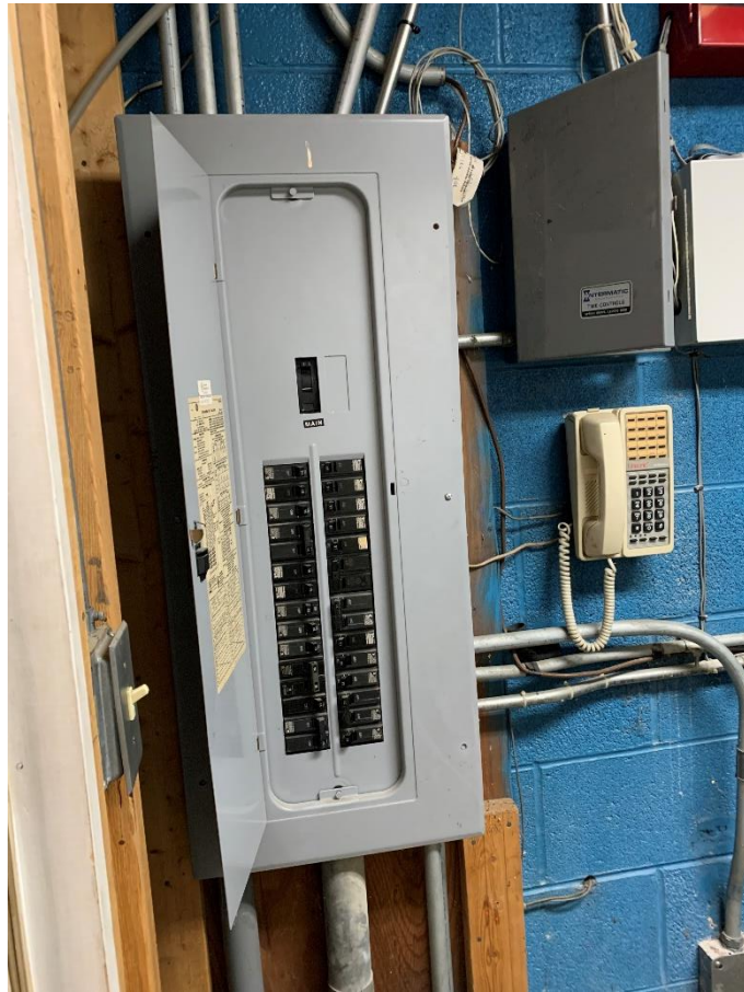
Figure 19 – Fire Training Building Main Service Panel
