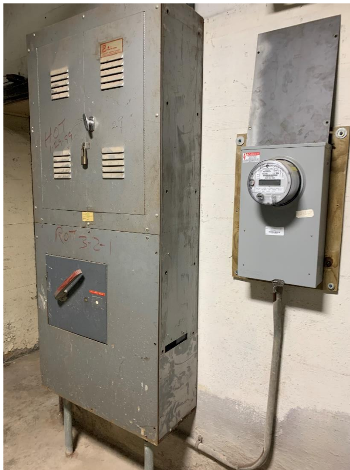
Figure 1 – Village Hall Main Service Switch and Meter
