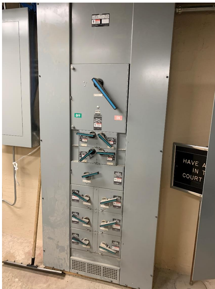
Figure 2 – Village Hall Main Service Panel
