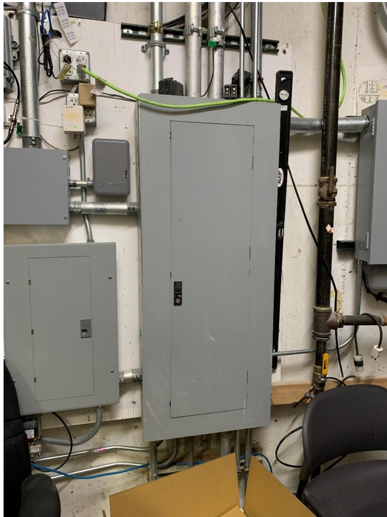
Figure 18 – Brian Carey Center Main Service Panel/Sub-Panel
