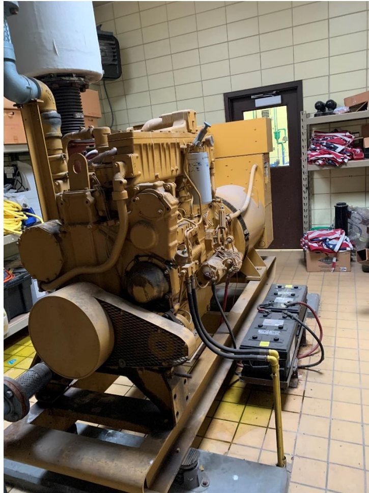
Figure 17 – Pump Station No. 2 Natural Gas Generator
