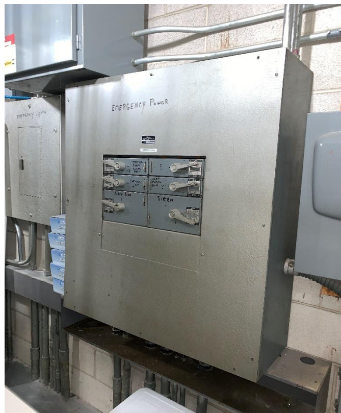
Figure 10 – Police Station Emergency Power Panel
