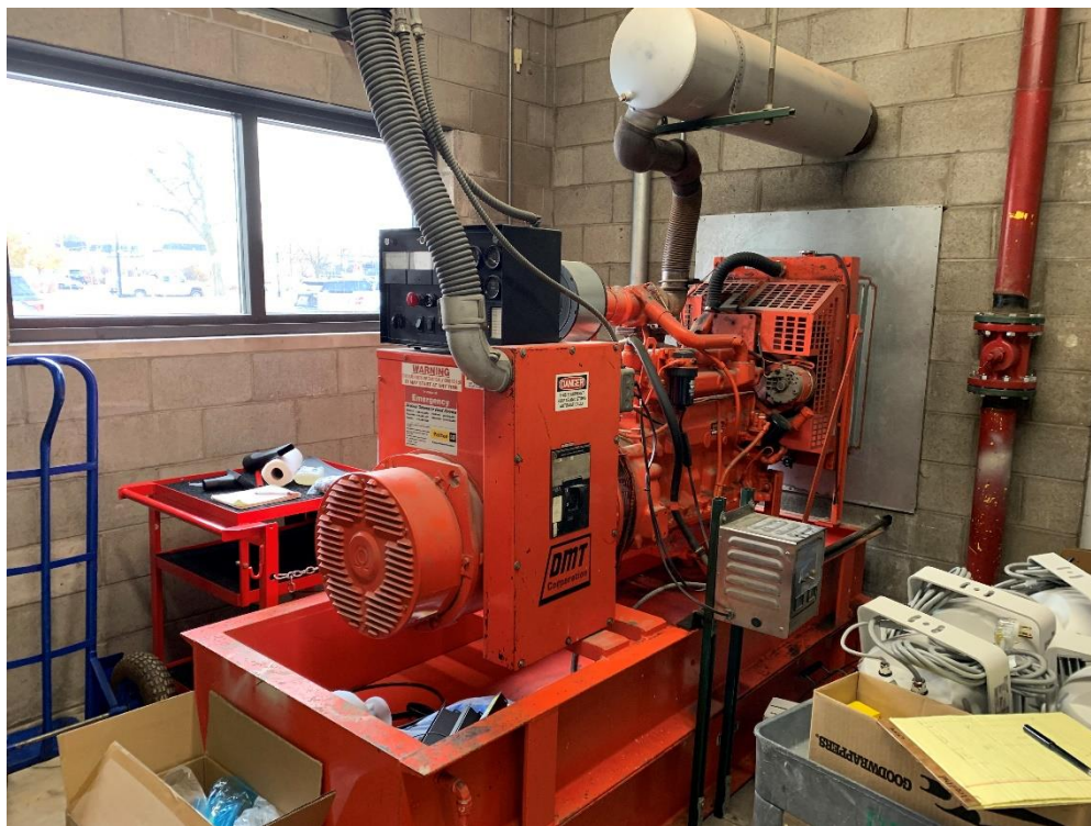
Figure 7 – Police/Fire/Village Hall Generator Set
