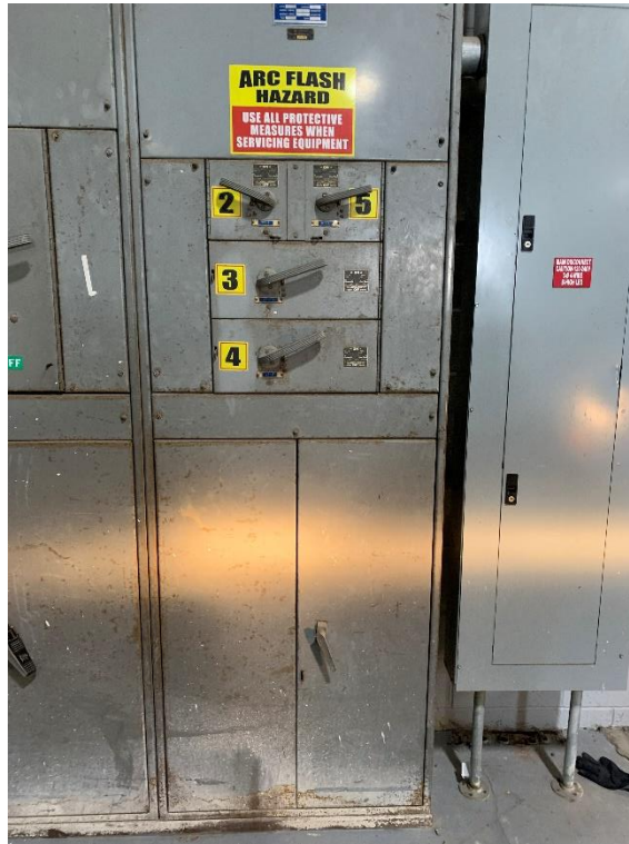
Figure 15 – Main Service Distribution Section No. 2
