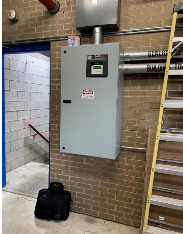
Figure 8 - Generator Automatic Transfer Switch
