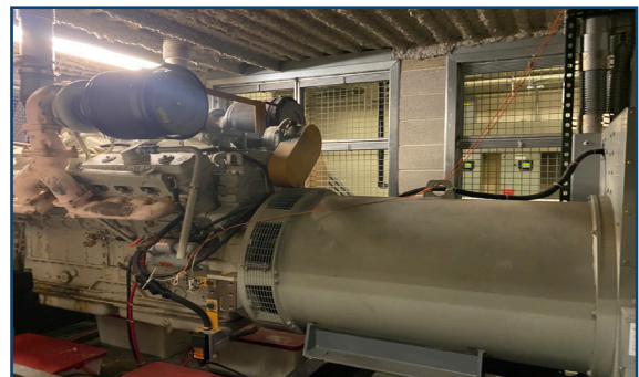
Existing Diesel Generator located inside the Richard J. Daley Center
