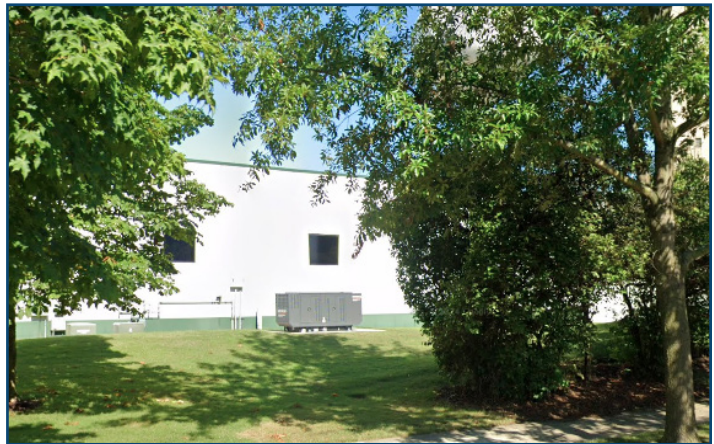
Homewood Flossmoor Generator
