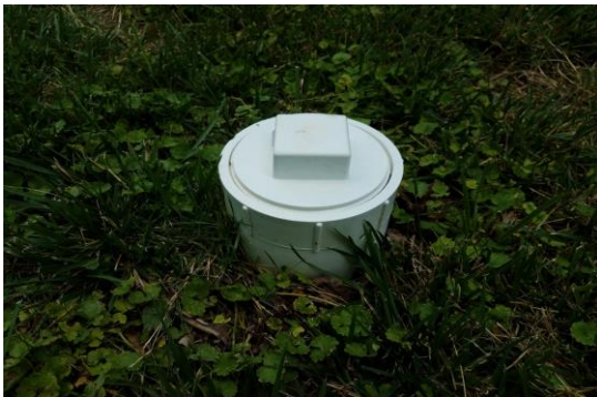
PVC Sewer Cleanout
