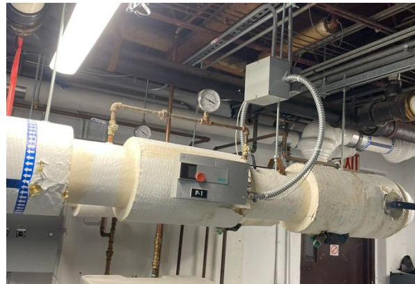
Police Department ground loop pumps
