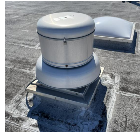
Typical roof mounted exhaust fan
