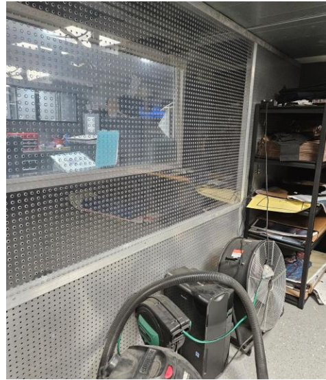
Shooting Range perforated supply air wall
