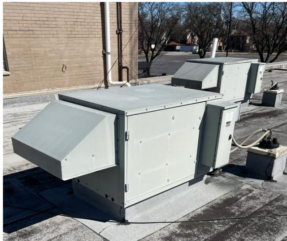
Police Department energy recovery ventilators
