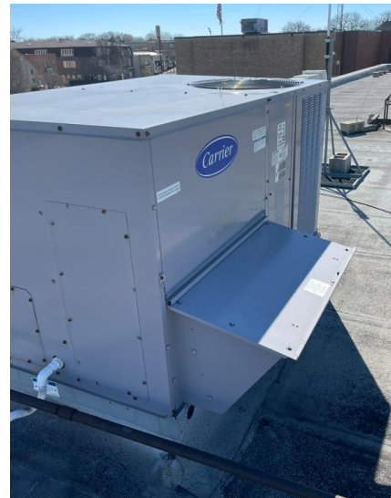
Fire Station dormitory rooftop unit
