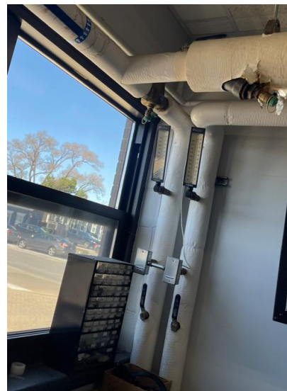
Piping to / from geothermal field (Fire Station)
