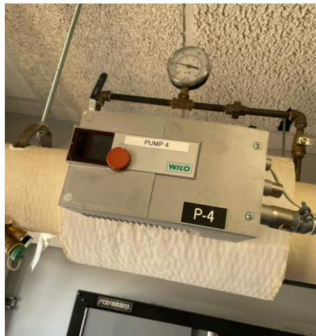
Fire Station ground pump
