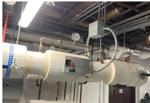
Police Department ground loop pumps
