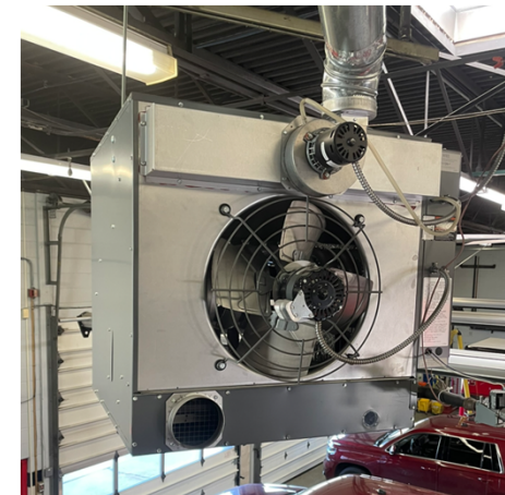
Typical gas-fired unit heater
