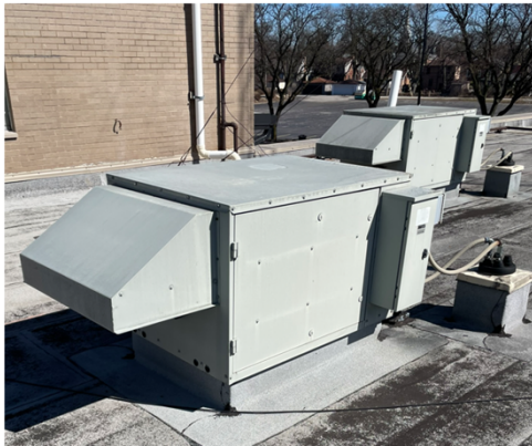
Police Department energy recovery ventilators
