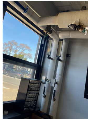
Piping to / from geothermal field (Fire Station)
