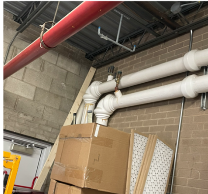
Piping to / from geothermal field (Police Department)
