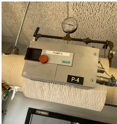
Fire Station ground pump
