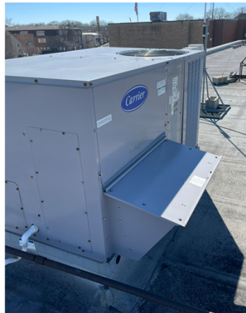
Fire Station dormitory rooftop unit
