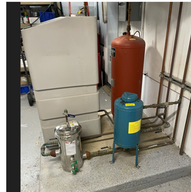
Police Station ground loop equipment (glycol feeder, expansion tank, pot feeder & side-stream filter)
