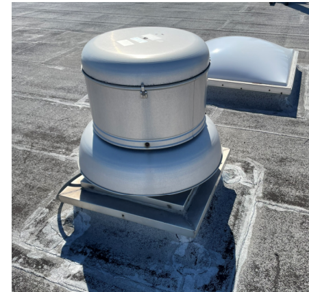
Typical roof mounted exhaust fan
