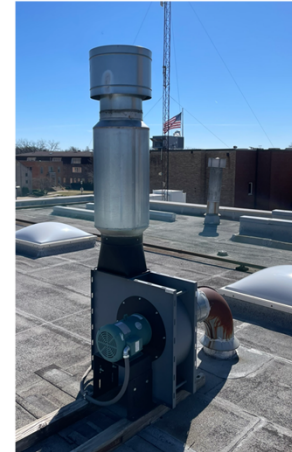
Apparatus Bay source-capture exhaust fan
