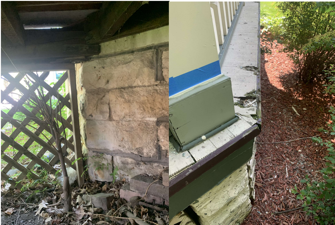
EXAMPLES OF ROTTING WOOD ELEMENTS
