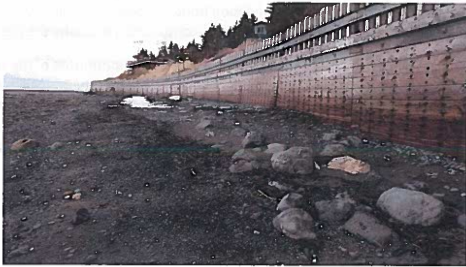
Figure 4- January 2019 Middle of Wall
