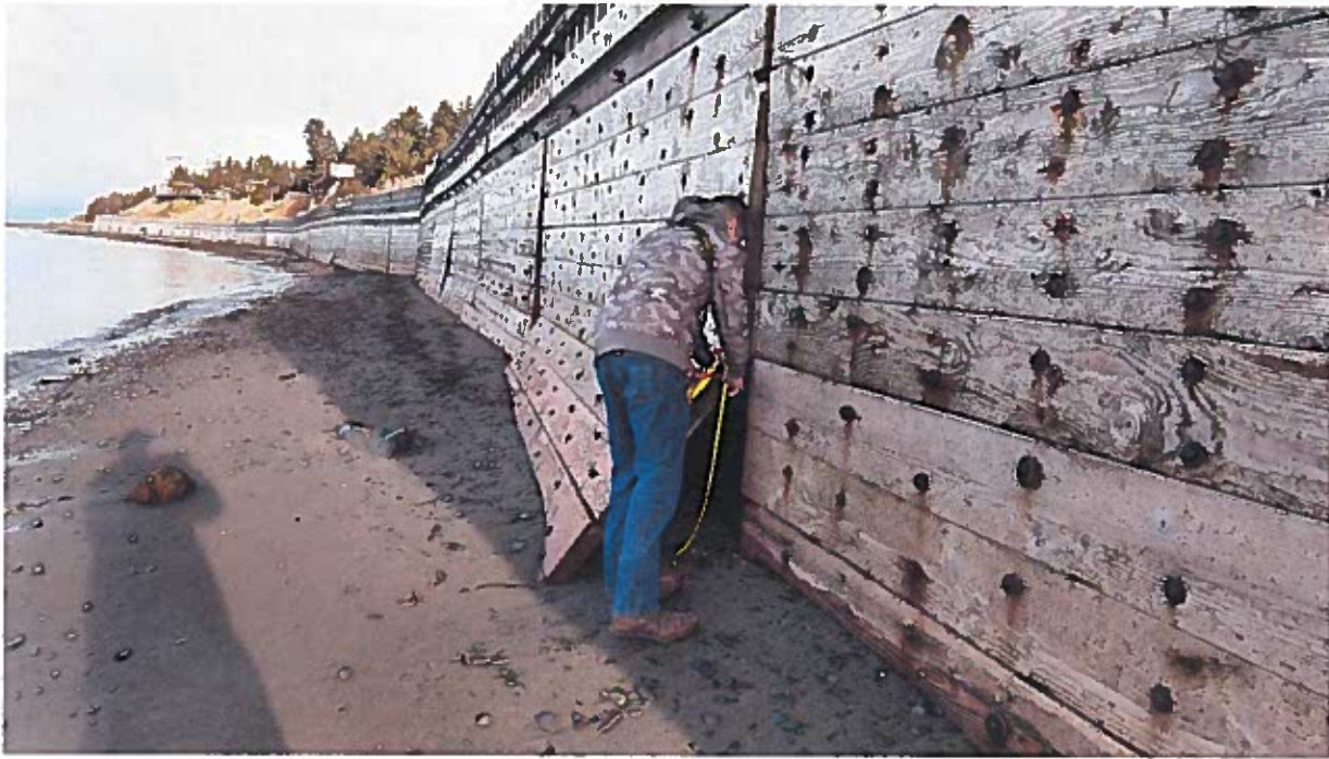
Figure 5- HDR, Inc. inspection of wall to assess damage in support of recommending potential long term improvements.
