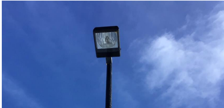
Metal Halide Pole Fixture at Lift #1
