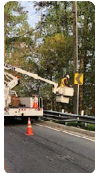
City Foot Traffic Street Electric & existing pole
