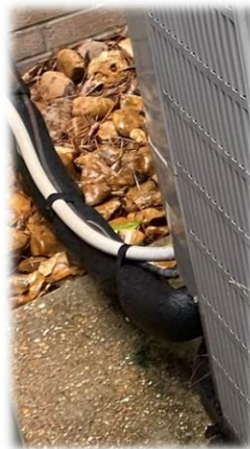
Figure 10. Well maintained insulation on refrigerant lines at the City Hall.
