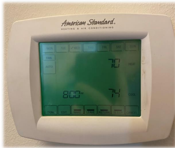
Figure 7. Programmable Thermostat schedule at the City Hall.
