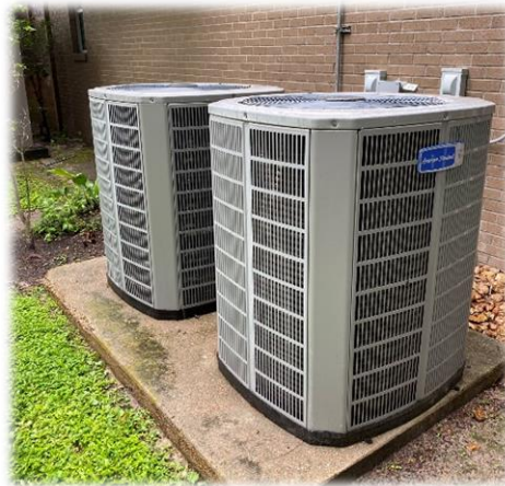
Figure 9. Hail guards on Split-DX units at the City Hall.
