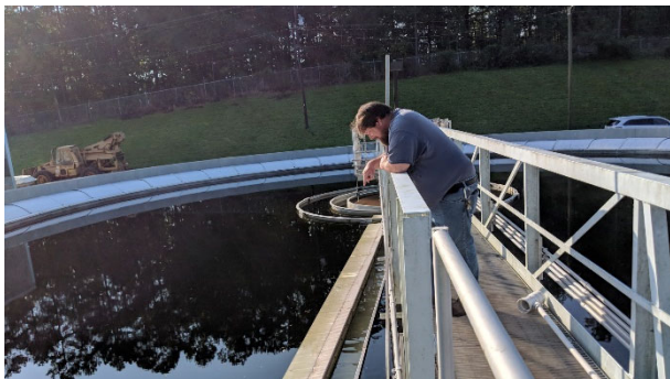
A utility mechanic inspects a mechanical arm on the Wastewater Treatment Plant's clarification tank, which sweeps the water surface of large organics and trash.
