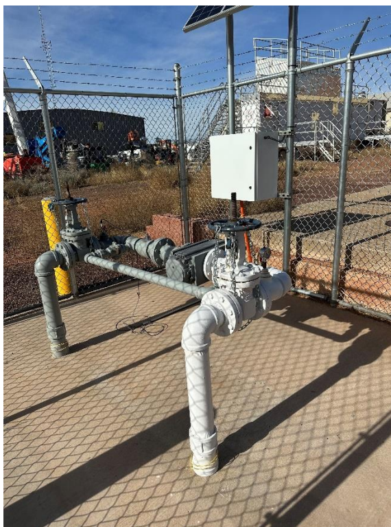
(Colorado City Natural Gas Gate Station)
