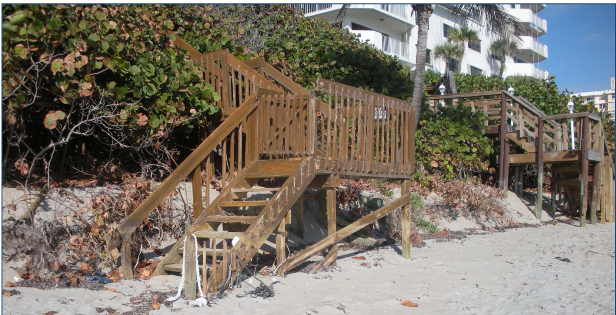
Photo 7. View of a scarped dune and beach erosion. Note that there is an approximate paint line on the staircase, which generally indicates a previous beach elevation and shows erosion of the beach. The missing handrail suggests recent damage from Hurricane Sandy.
