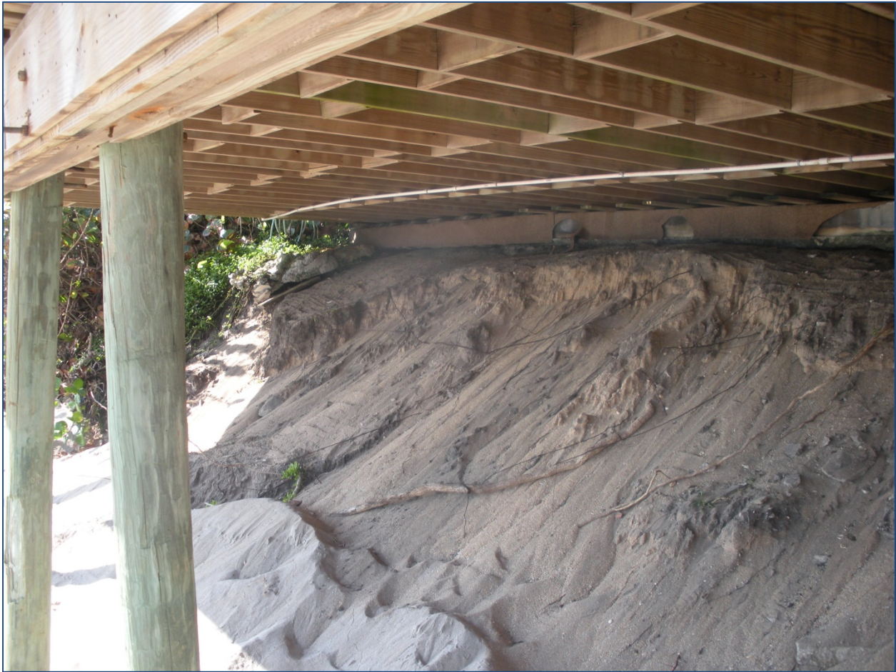
Photo 8. Deflation of the dune underneath the deck at 4513 S Ocean Blvd, likely as a result of Hurricane Sandy.
