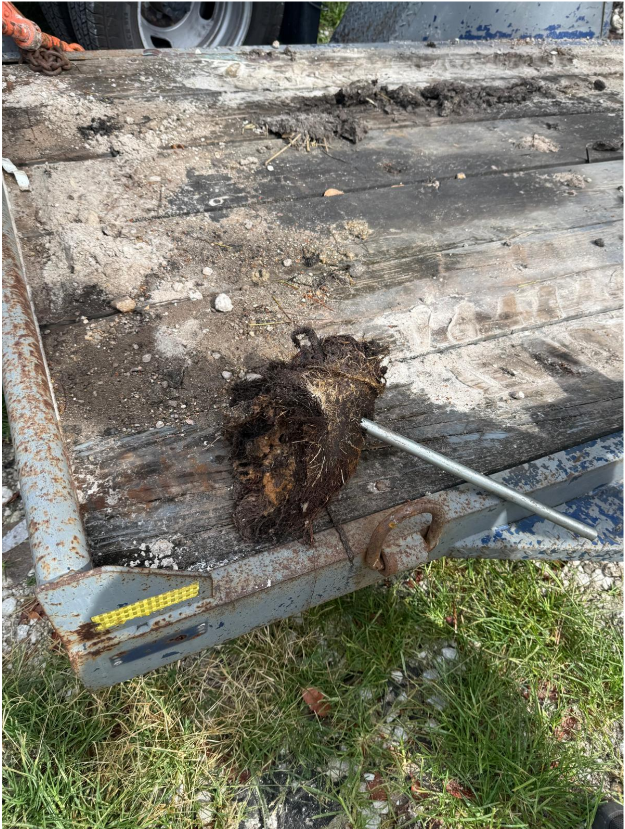
Photo of FPL's leaking Transformer and Roots in City Sewer line.
