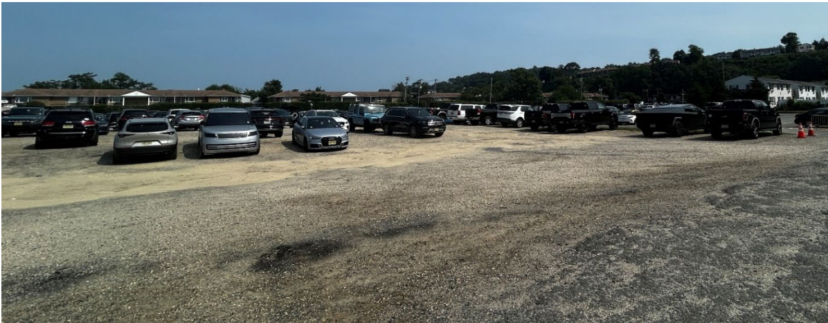
Combination of gravel, sand, and asphalt within the main parking lot.
