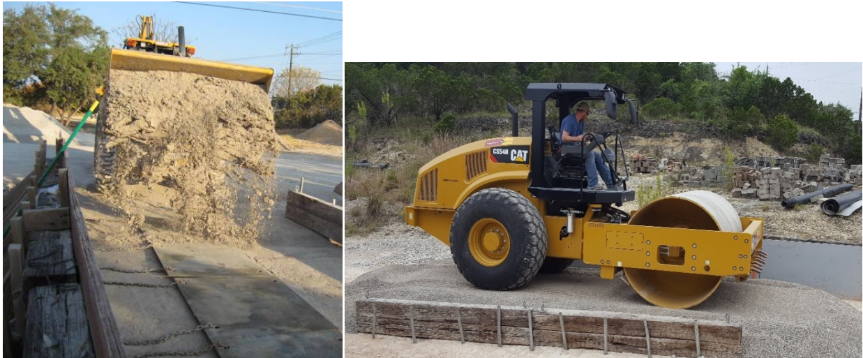
Figure D-1. Lifting Plates positioned between ties and covered with first lift of compacted soil/aggregate.
