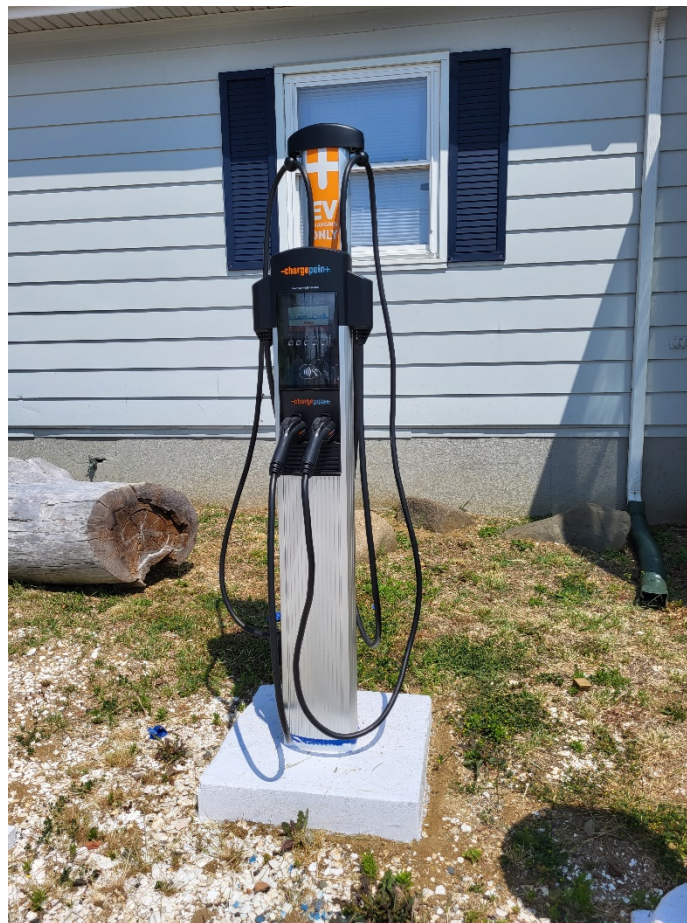
Photo 2: Existing EV infrastructure
