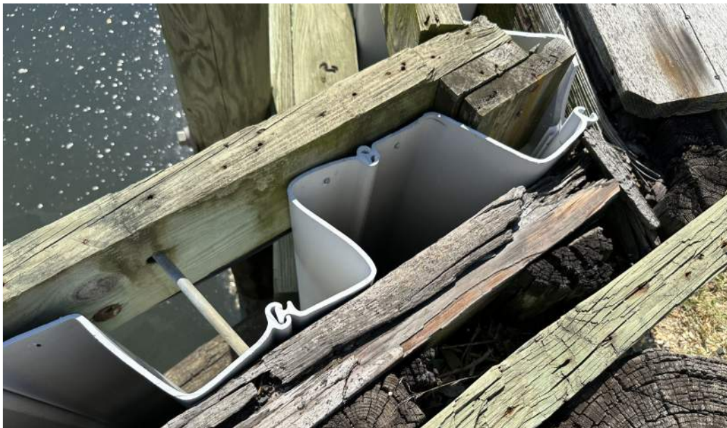
Photo 25: Section C, Westerly Bulkhead, Viewed of Crushed Sheet Pile
