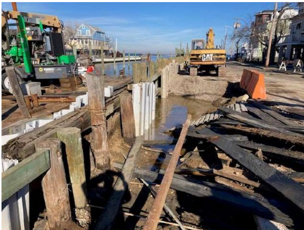
Erosion right up to roadway
