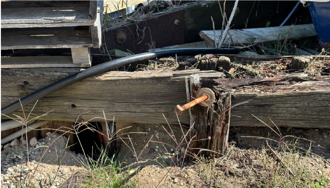
Southernly Bulkhead, Fastener and metal sheetpile bulkhead condition (From Colliers Engineering and Design's Report dated November 4, 2024)
