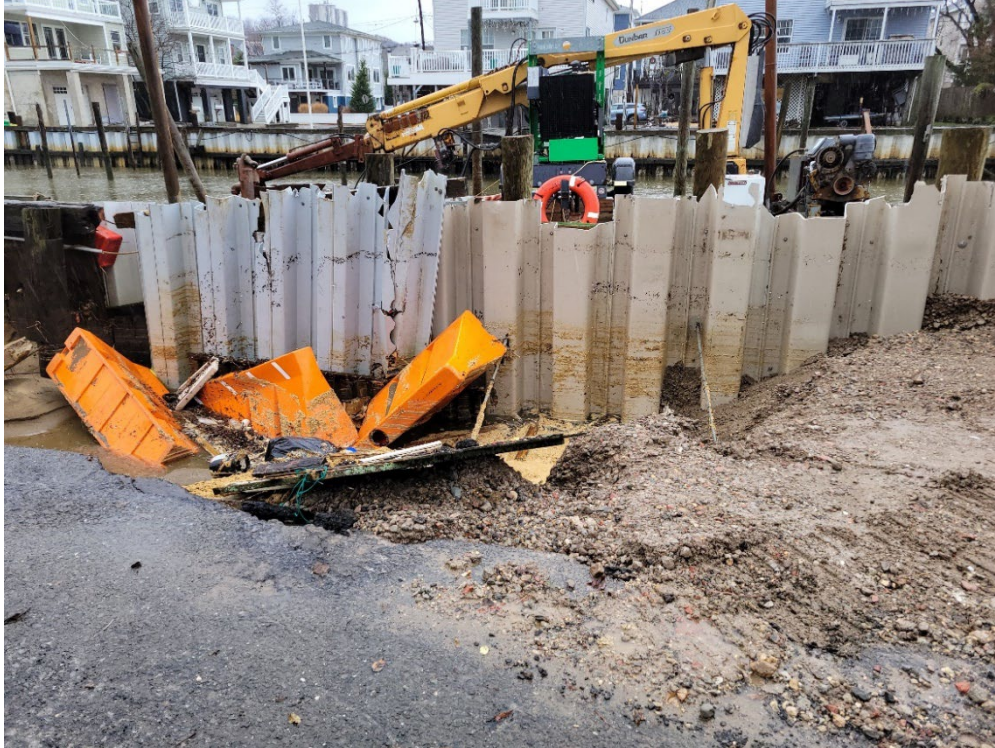
Photo depicting poor condition of the bulkhead along Washington Avenue (December 2022) (Provided by Michael Muscillo)
