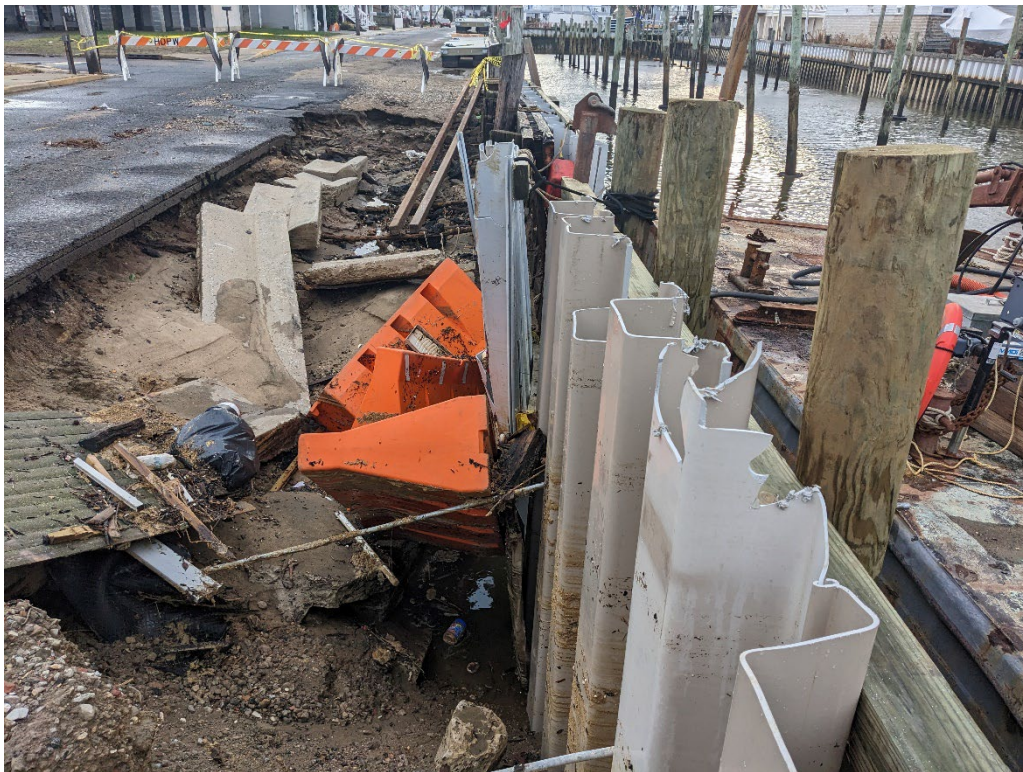
Damage to the Washington Avenue Right-of-Way (12-23-2022)(Provided by William Brunt)
