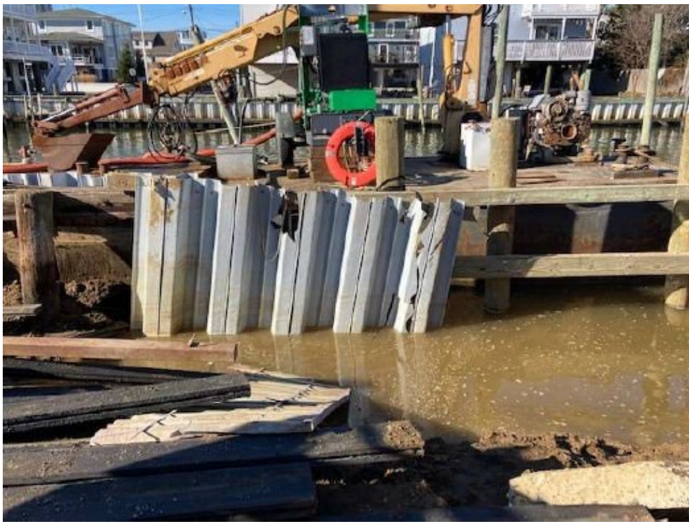
Road sub-base eroded into the cove (From Colliers Engineering and Design's Letter dated January 9, 2023)
