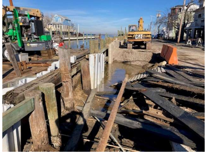
Erosion right up to roadway
