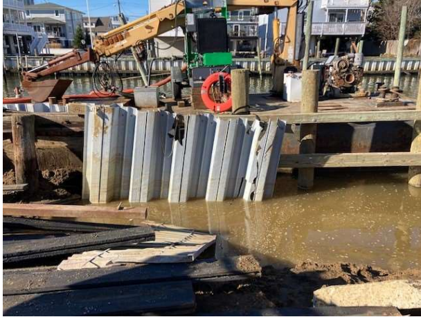
Road sub-base is eroded into Cove
