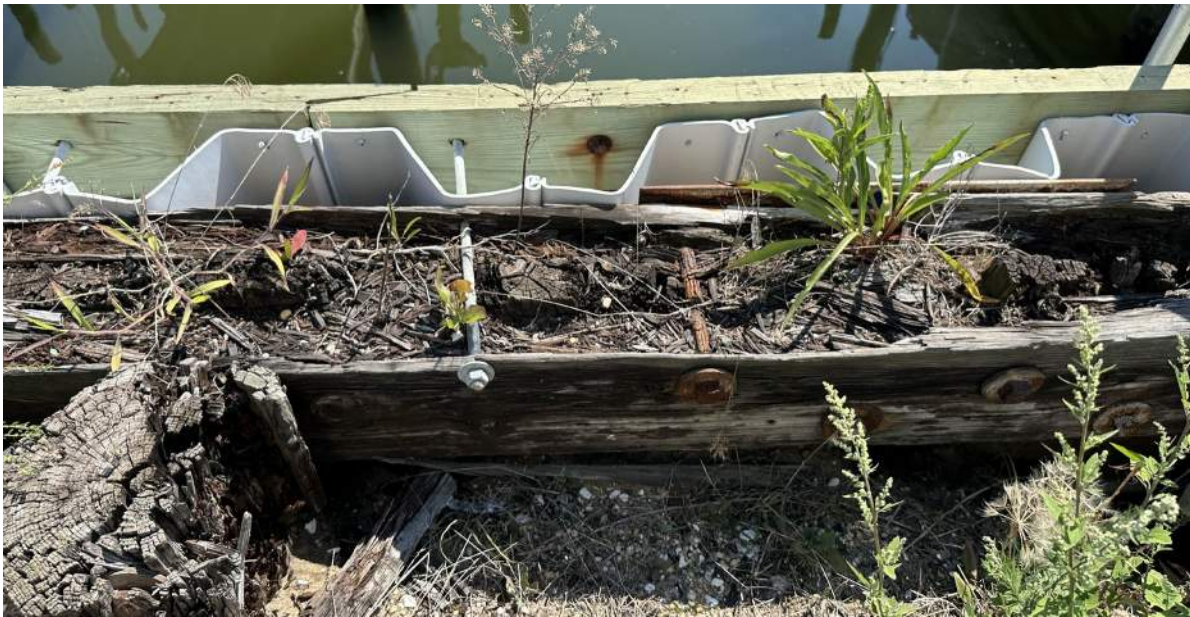
Photo 26: Section C, Westerly Bulkhead, Deteriorated Timber Elements & Fasteners, View 1
