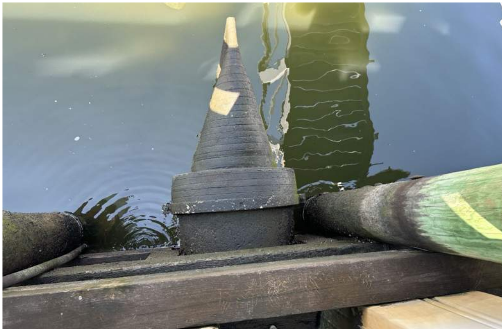
Photo 11: Section A , Easternly Bulkhead, Outfall Pipe with Outfall Backflow Preventer (Tideflex)
