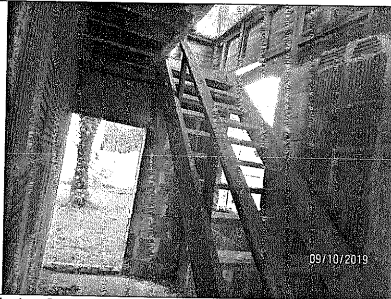
Photo No.: 7 (facing South) Description: View of partially damaged staircase located at northern face of building.
