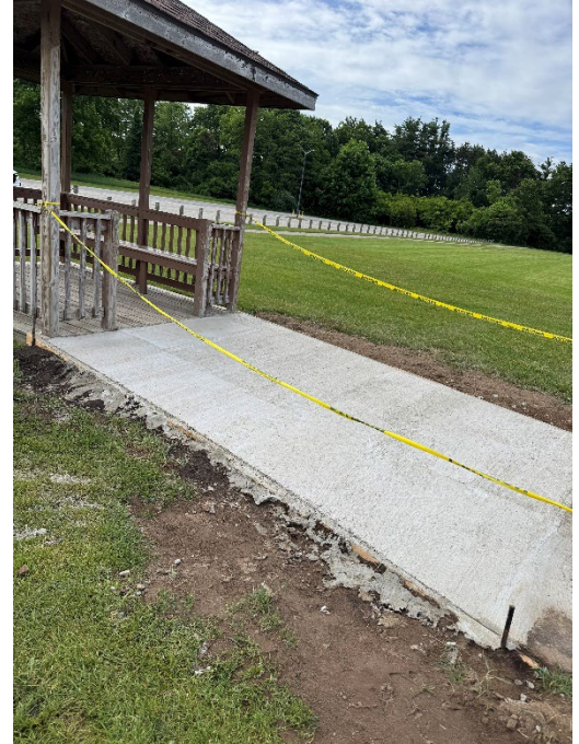
Figure 4- Gazebo Pathway – This structure needs stain and minor repair. Suggest Brown Stain, with Dark Green Trim like Adult Workout.
