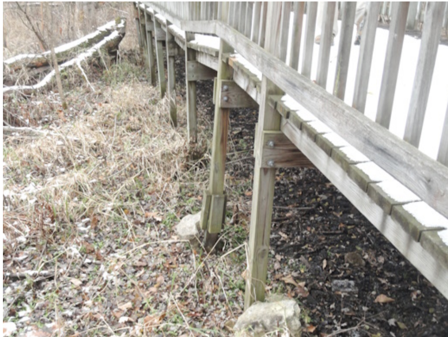
Figure 6: Existing post repairs with heaved concrete surrounds
