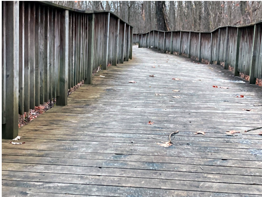
Figure 4: Humps and excessive cross-slope
