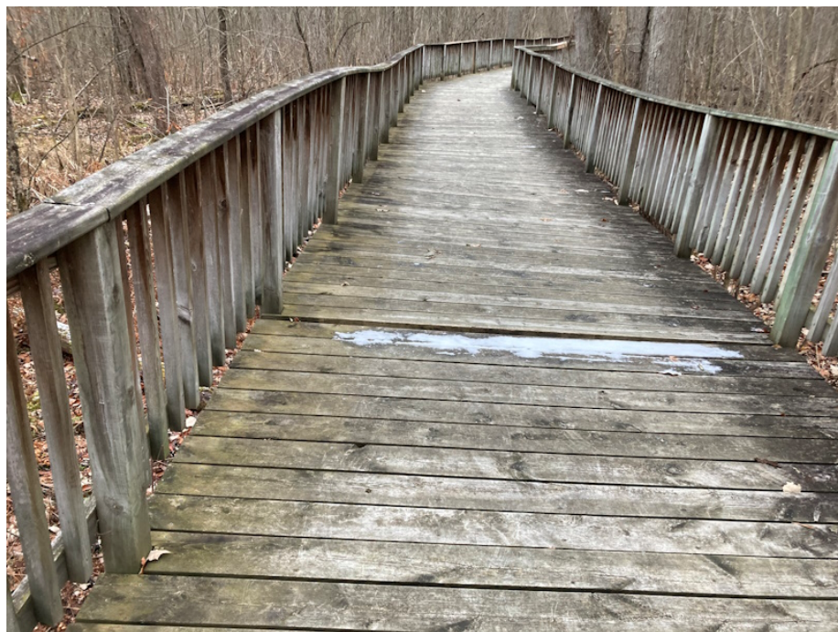
Figure 3: Trip hazard at raised deck board
