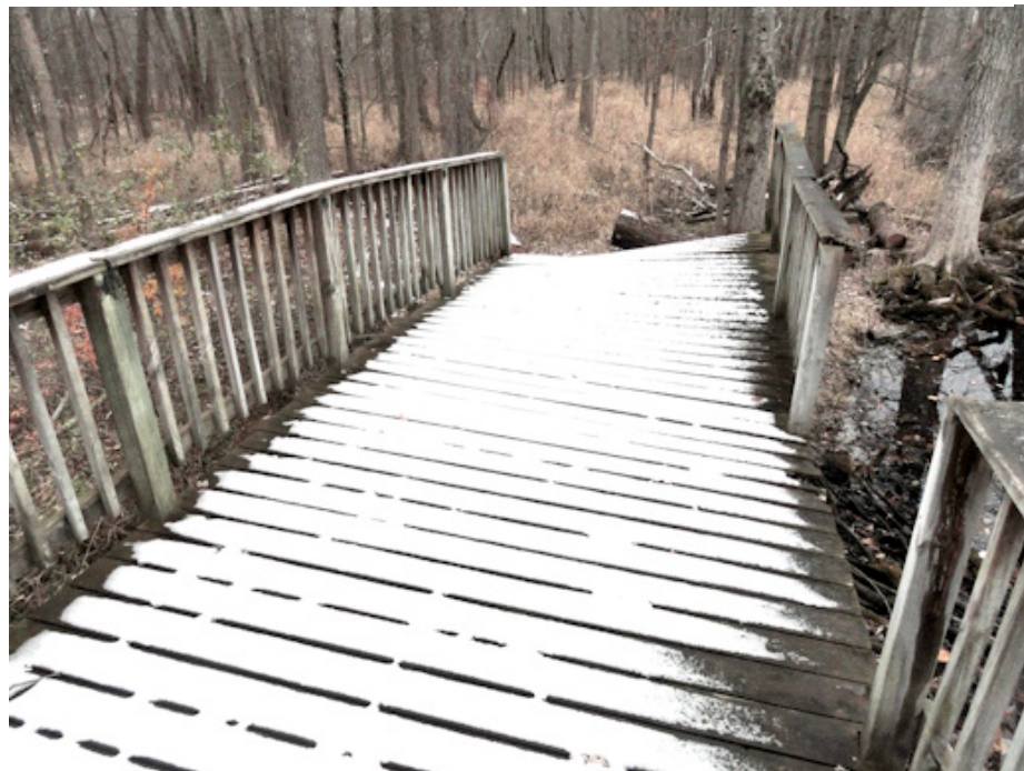
Figure 5: Collapsed end at river
