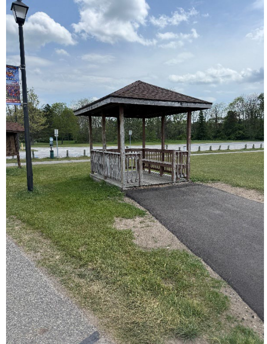
Figure 4- Gazebo Pathway (Transition must be flush with surface) – This structure needs stain and minor repair. Suggest Brown Stain, with Dark Green Trim like Adult Workout.
