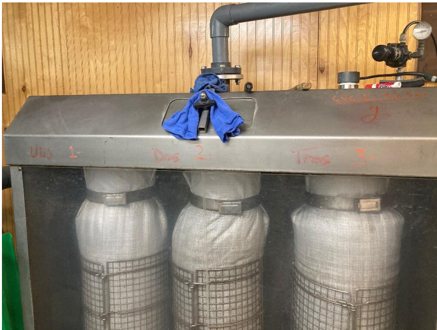
Figure 7. The sludge bagger at Bartlett Cove wastewater treatment facility.
