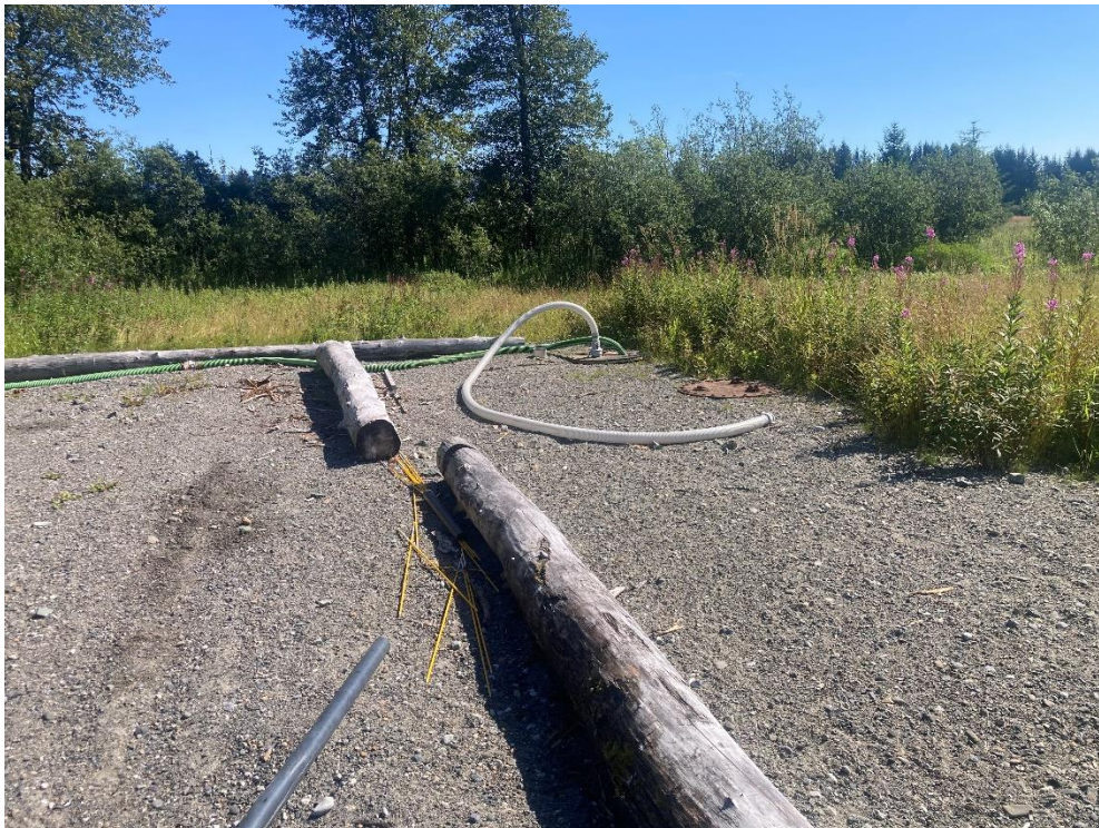
Figure 3. Caps of one of the septage holding tanks
