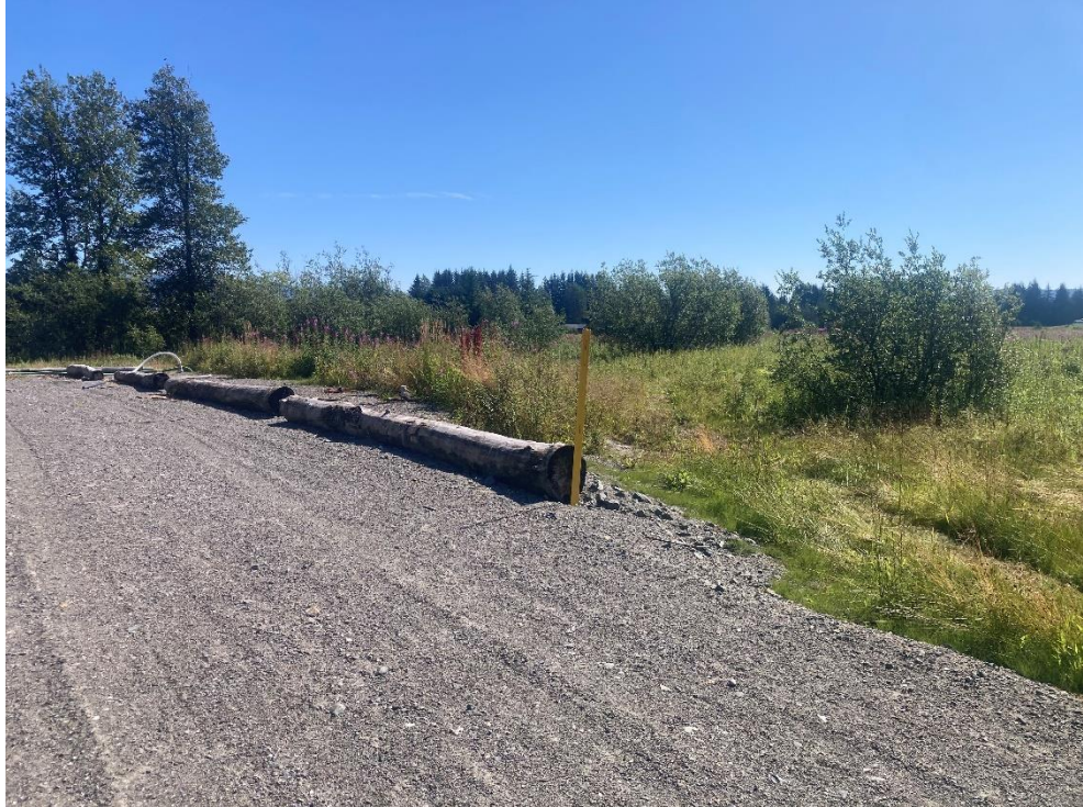
Figure 5. Location of the septage holding tanks
