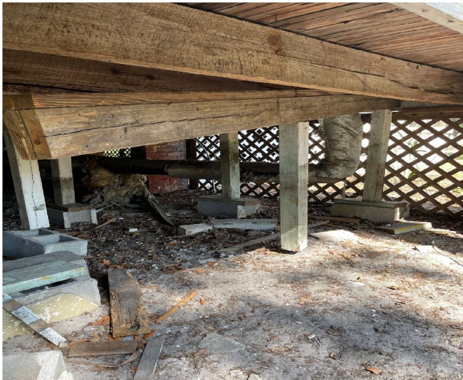
Photo 9: Enclosed Porch Floor Framing – Previous Repair/Unsupported Beam
