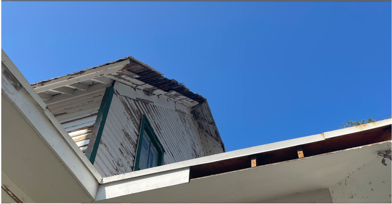
Photo 4: Deteriorated Boards Supporting Metal Roof
