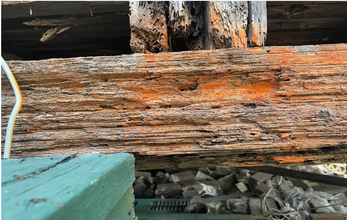
Photo 6: Rear Addition – Deteriorated Perimeter Beam
