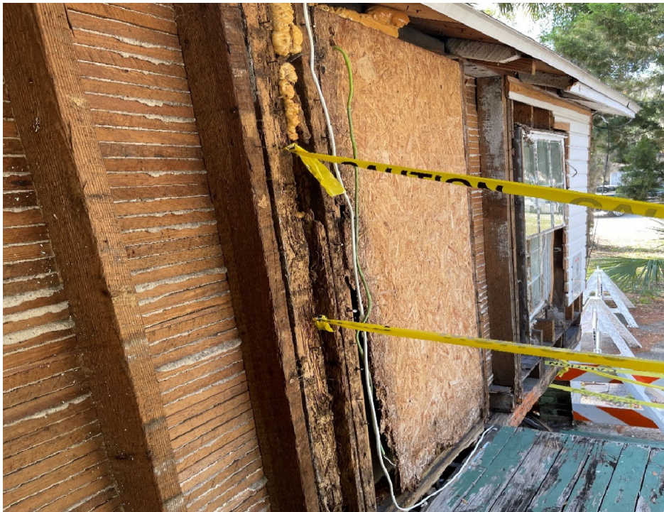
Photo 7: Rear Addition – Damaged Studs
