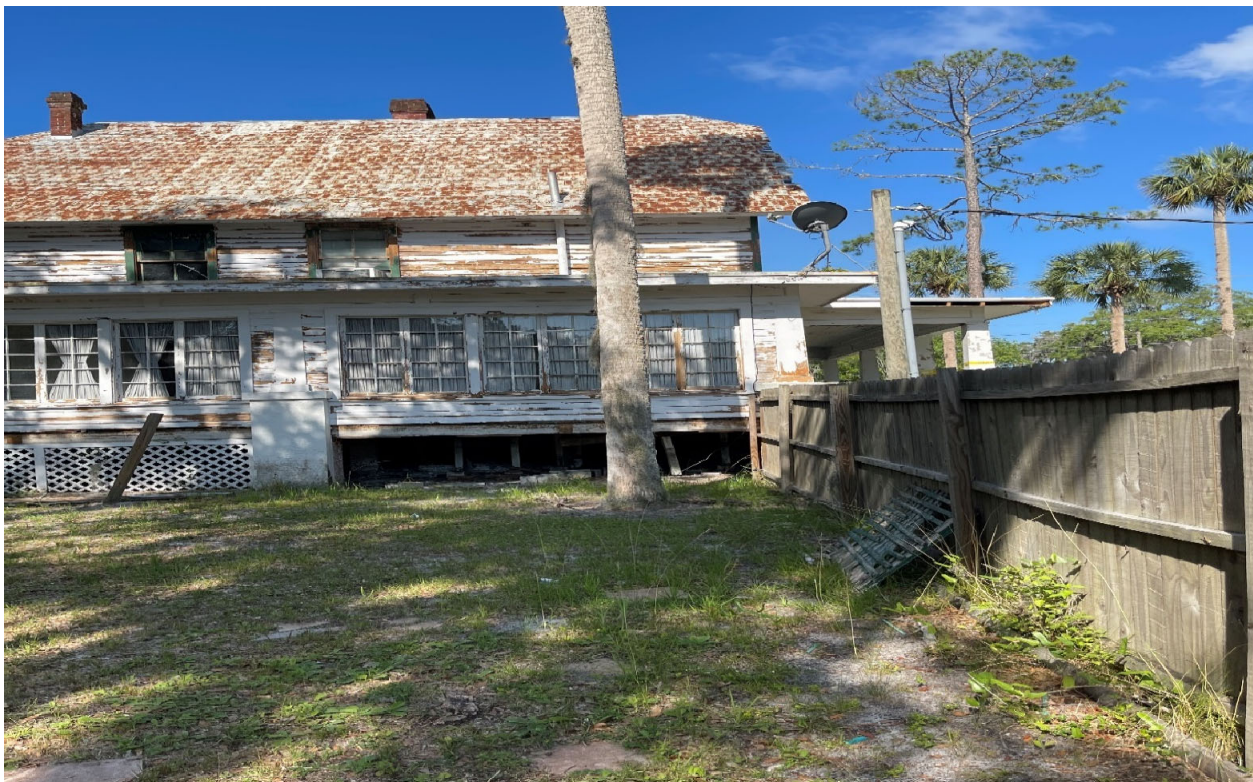
Photo 2: Left Side Main Home/Enclosed Porch – Note Rust to Metal Roofing
