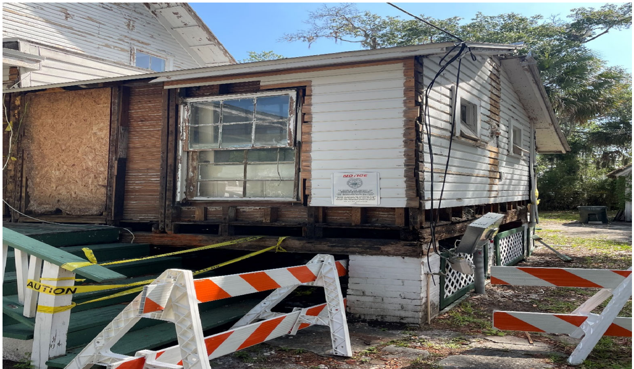
Photo 5: Dilapidated Rear Addition
