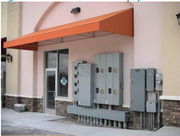
Prohibited (utilities facing street)
