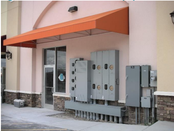
Prohibited (utilities facing street)
