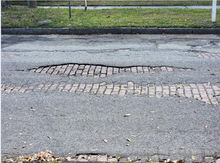
Figure 5. Road Disrepair, Walnut St
