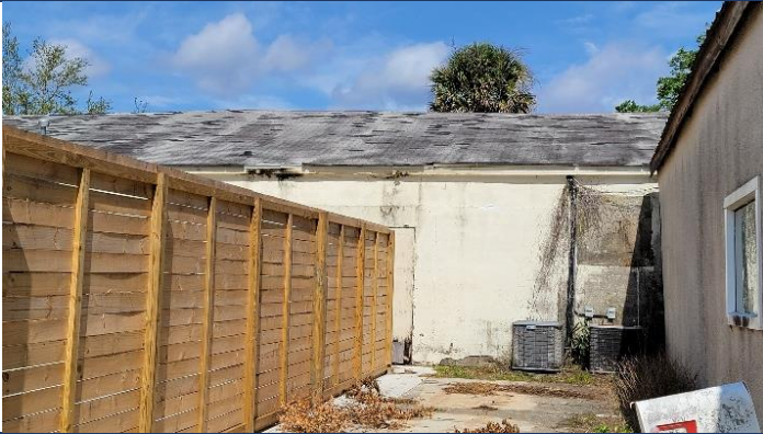
Figure 15. Unsafe, Boarded Openings, 115 N Magnolia Ave
