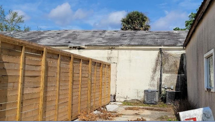
Figure 15. Unsafe, Boarded Openings, 115 N Magnolia Ave
