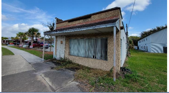
Figure 16. Unsafe and unsanitary, Openings / Junk Storage, 115 N Magnolia
