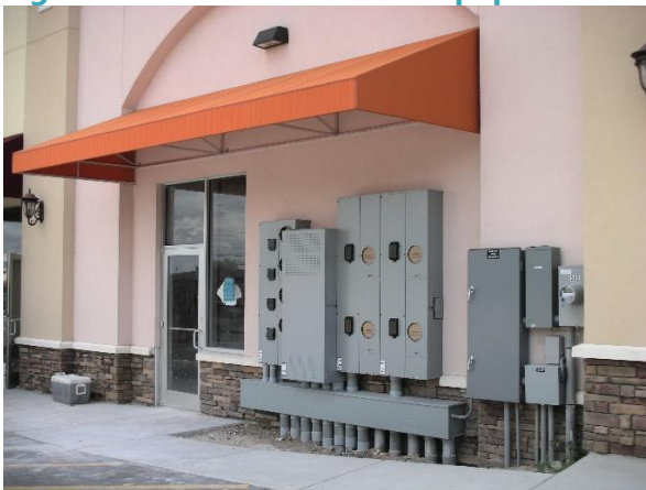
Prohibited (utilities facing street)
