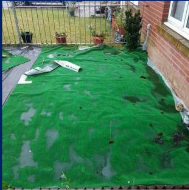
Site Drainage Issues
