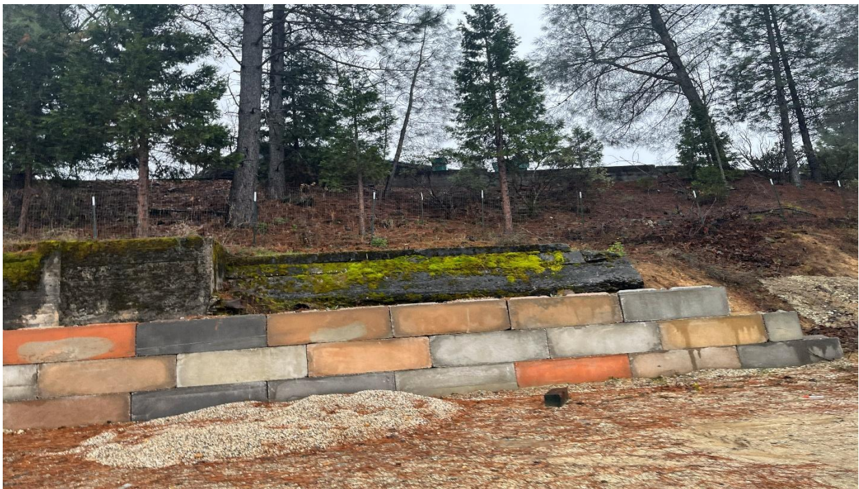
Photo 4: Photo looking south from the Project area with an existing retaining wall and some pine trees upslope outside of the Project area. Trees are outside Project fenceline.
