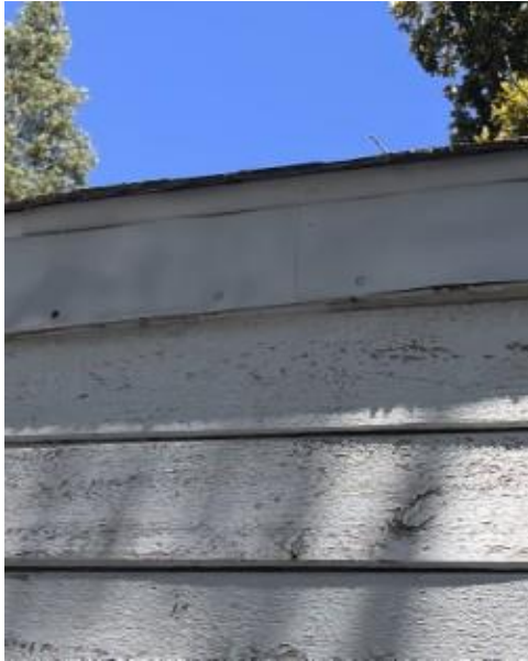
Figure 6 (left) – View of existing roof edge. Proposed material image below (left) indicates a 2-inch drip edge made of galvanized edge flashing, layered over a 6-inch galvanized flat flashing; intent is to replicate existing flashing on primary home roofline.
