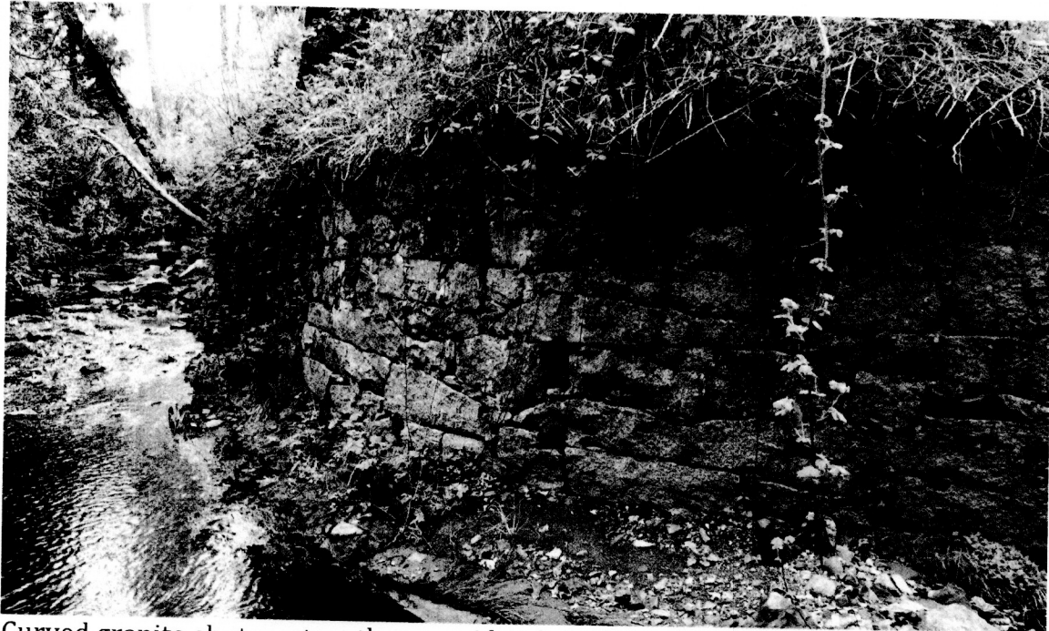
Curved granite abutment on the east side of Wolf creek viewed from the western bank. When the railroad grade constructed in 1875 followed the route of the creek with wooden approaches and dirt fill. Subsequent winter storm damage led the railroad to reinforce the trestle abutments with granite here.
