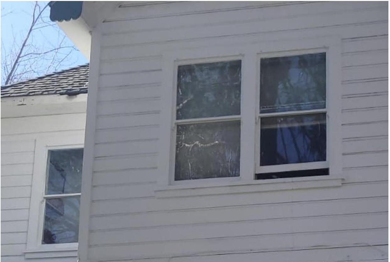
Image of replaced windows from applicant (upper level windows)
