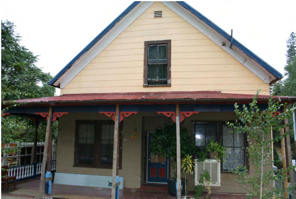
Close-up of the front facade of the residence. Note the bracing on the porch columns.
