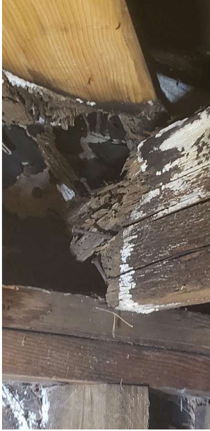
Figure 1- Deteriorated Floor Joist
