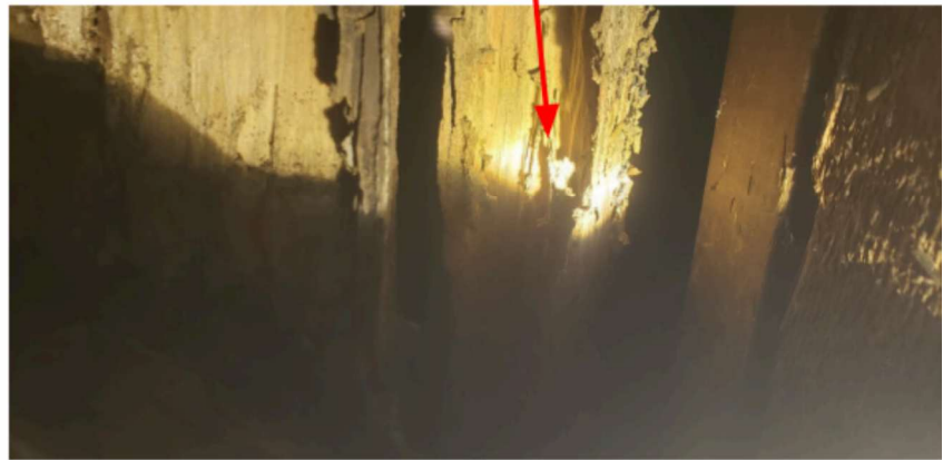
Figure 4- Decayed wood in southernmost column
