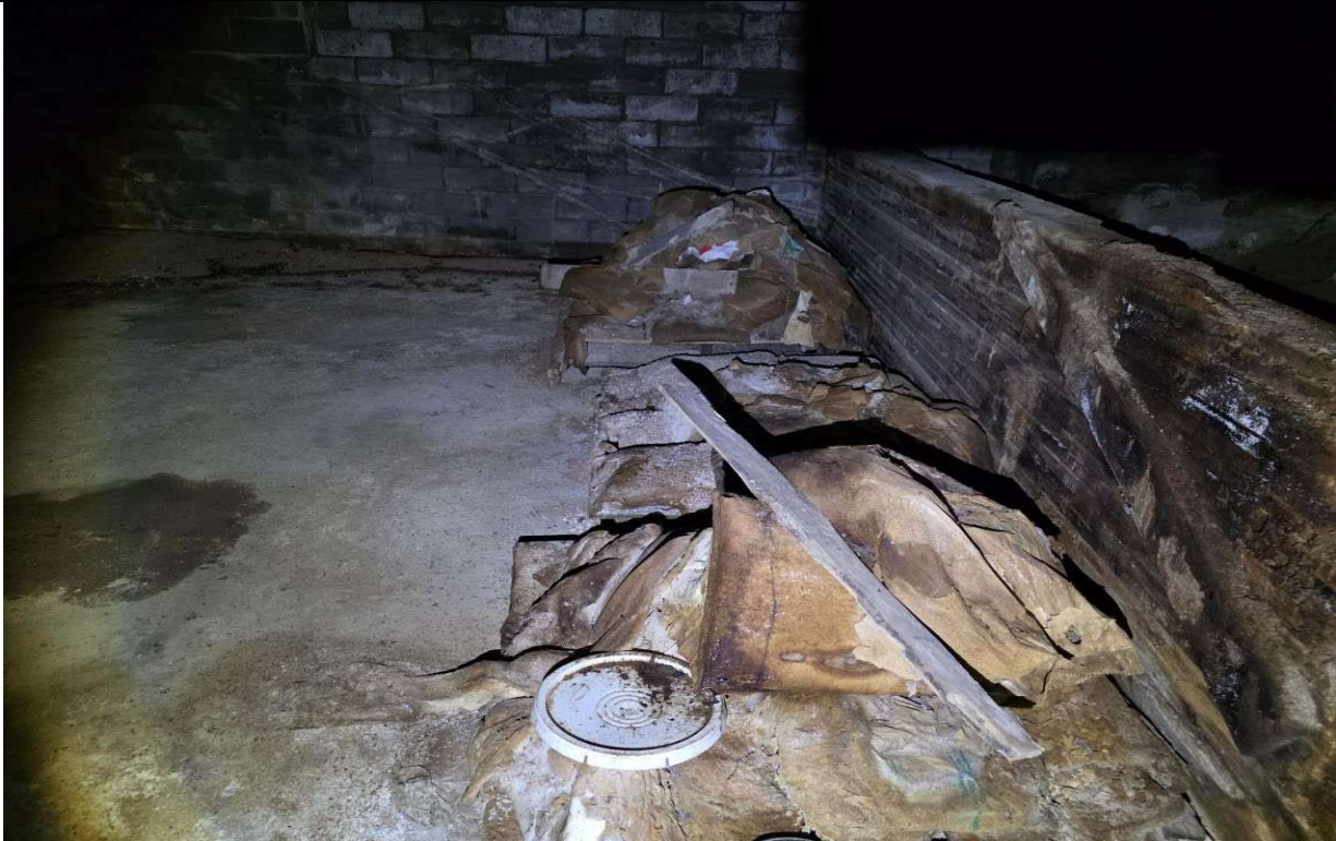
Photograph 33 Date: April 14 th , 2026 Direction: North Subject: Approximately 5000lbs of unidentified fertilizer in the northwest portion of the Site building's basement bulk storage area.
