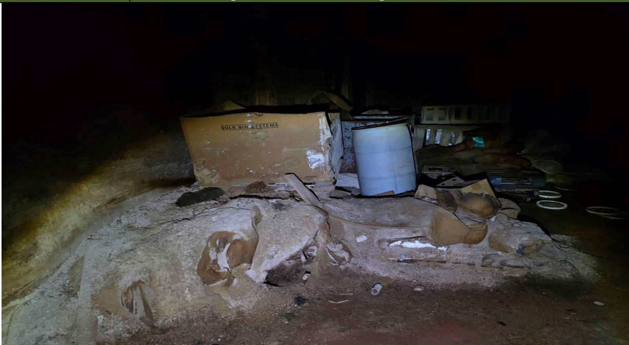
Photograph 36 Date: April 14 th , 2026 Direction: North Subject: Approximately 5000lbs of unidentified fertilizer and 5 drums half full of unidentified liquid in the northern portion of the Site building's basement bulk storage area.
